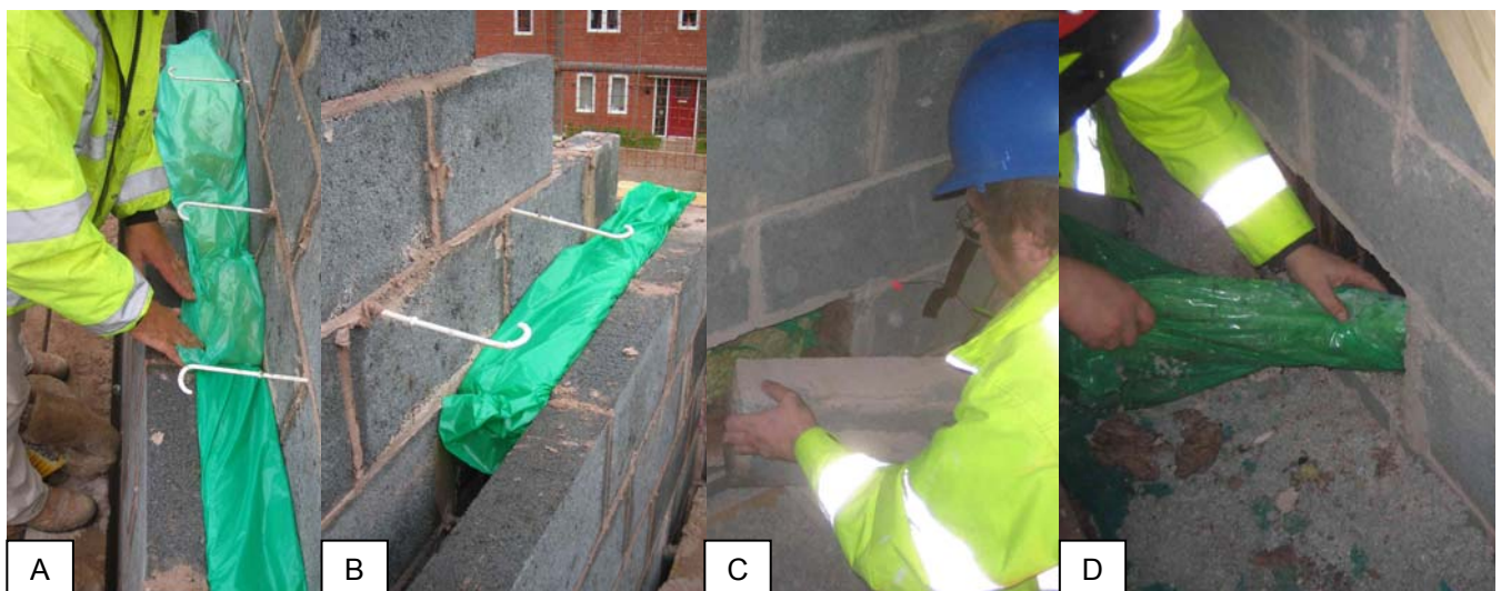
Figure 39 – Horizontal Cavity Sock Being Inserted into Party Wall Cavity during Construction (A,B) and then Being Removed again Halfway through the Coheating Test (C,D)
