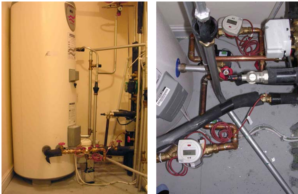
Figure 59 – Heat Meter Installation in Cylinder Cupboard
