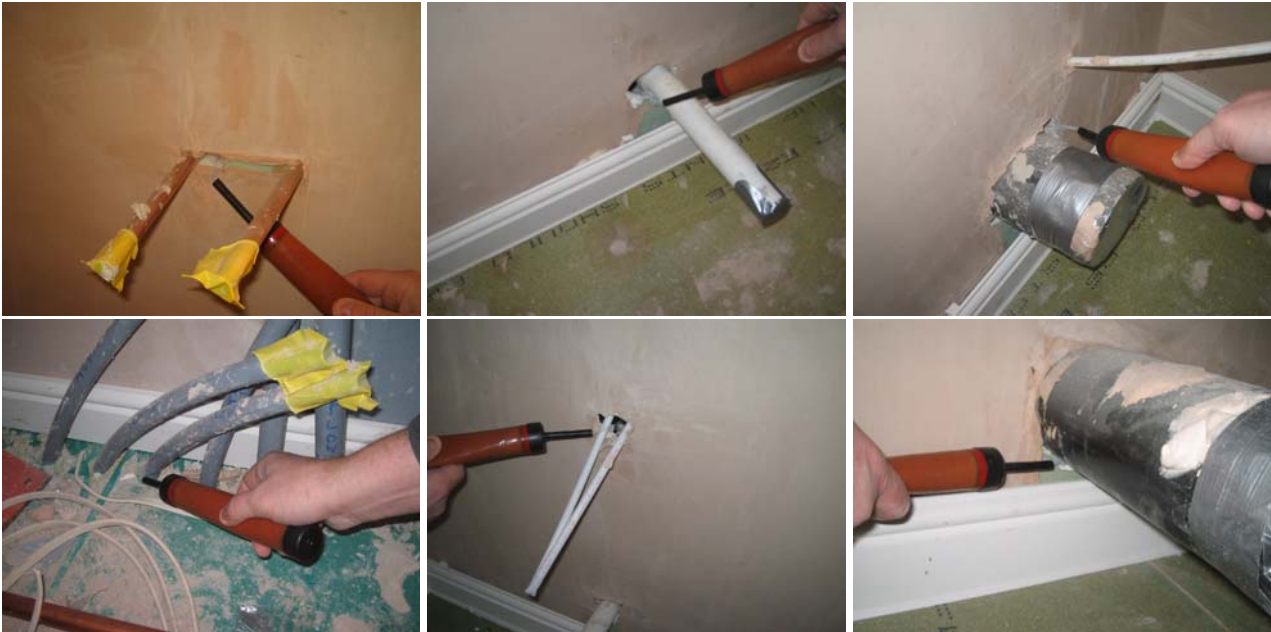
Figure 1.9 First floor plumbing penetrations in the bathroom, cylinder cupboard and en-suite.
