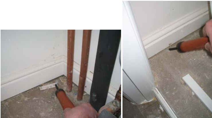
Figure 7.19 Air movement through unsealed gaps around the platform floor of the cylinder cupboard.
