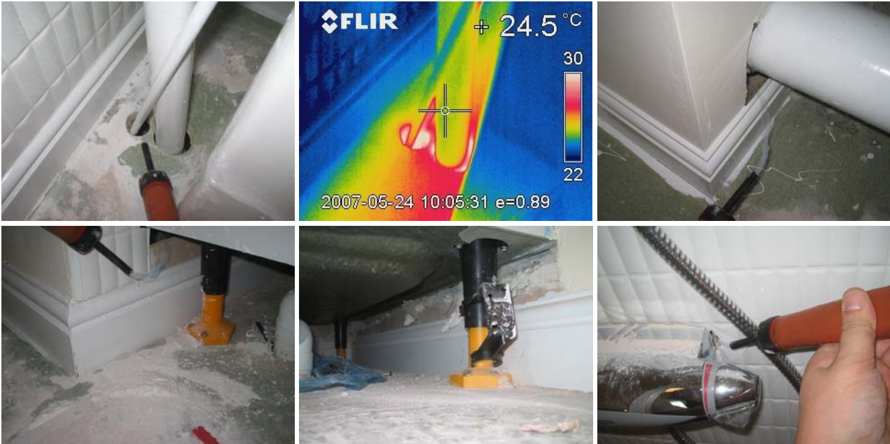
Figure 11.16 Unsealed plumbing penetrations on the 2 nd floor; into the intermediate floor, into the front en-suite service void, under the shower tray and around the shower control.
