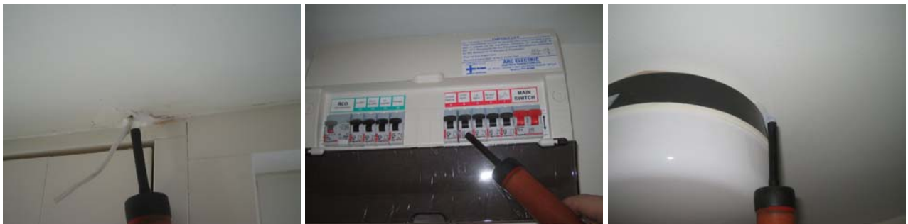
Figure 7.23 Air leakage around inadequately sealed electrical penetrations, including all the bathroom, ensuite and downstairs WC ceiling-mounted light fittings.
