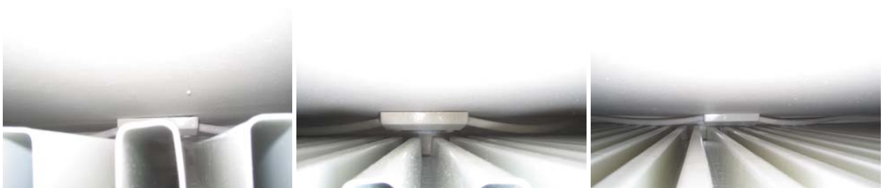
Figure 9.20 At all radiator pipework some air leakage was observed, with no apparent patterns between rate of leakage and position of radiator.
