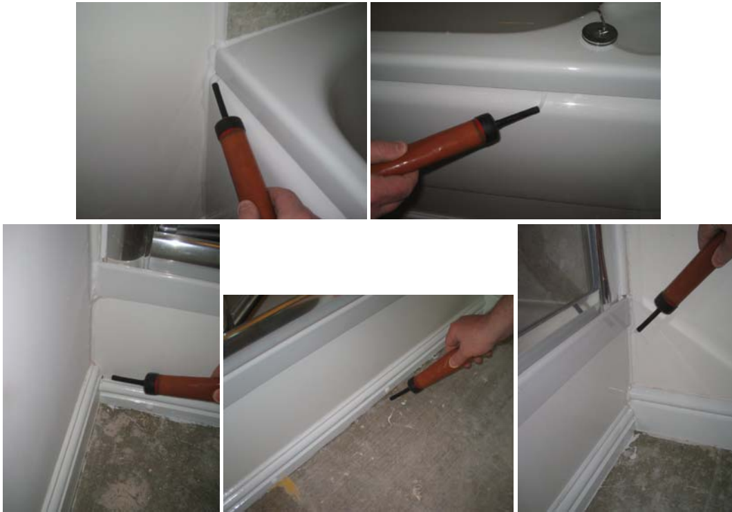
Figure 7.21 Points of air leakage around the bath panel and around the shower tray fascias.
