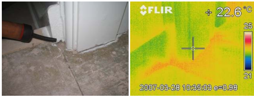
Figure 12.5 Air leakage at the junction of the 1 st intermediate floor with the stairs.
