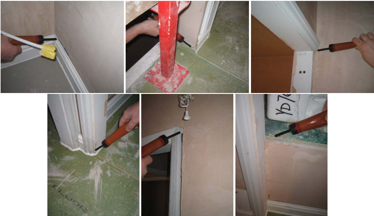
Figure 1.10 Air movement around skirting boards in the downstairs WC and landing, around architrave on the first floor in bedrooms and bathroom, and around the cylinder cupboard floor.
