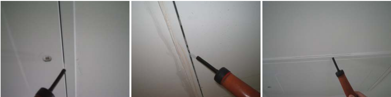
Figure 7.24 Air movement into the loft between the loft trap and door and at the junction of the loft hatch and bedroom ceiling.
