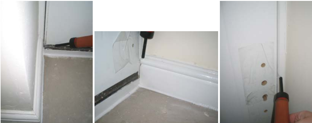
Figure 9.10 Air leakage around the back door
