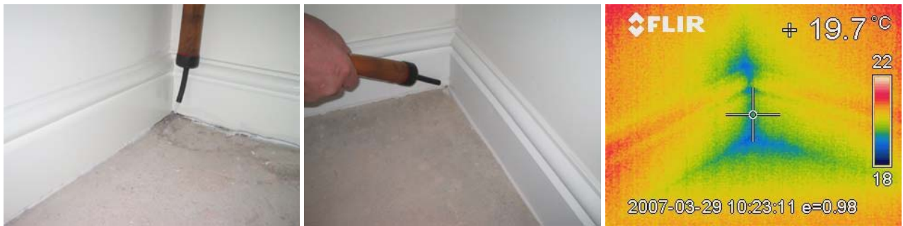
Figure 13.2 Ground floor room corners.
