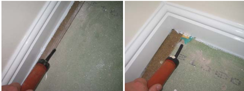
Figure 11.5 Air movement into the 1 st floor void through gaps in the flooring panels.
