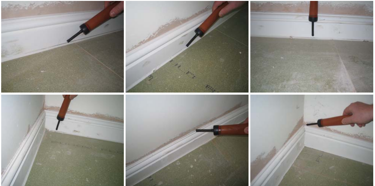
Figure 8.11 Air leakage detected at junctions of the intermediate floor with internal, external and separating walls where the sealant had failed and at shrinkage cracks above the skirting boards.
