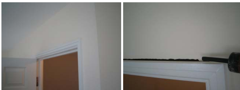
Figure 9.8 Air leakage was detected above a 2 nd floor internal door frame in the rear bedroom, where the unsealed gap was hidden by the architrave.
