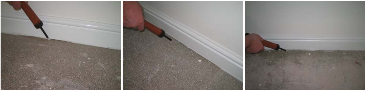
Figure 7.18 Air leakage around the second floor perimeter through gaps in the sealant in both bedrooms.
