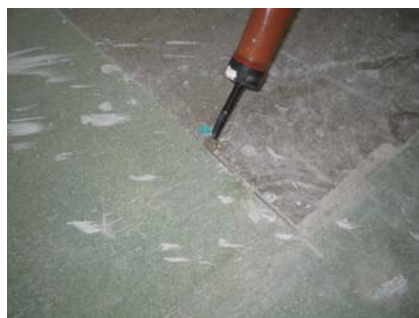
Figure 10.5 Air movement into the 1 st floor void through gaps around repairs to the floor in the lounge.
