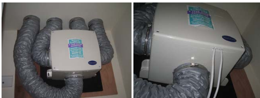
Figure 14.2 The MEV unit as when the initial pressurisation test was performed and with the additional wiring added by the time of the re-test.
