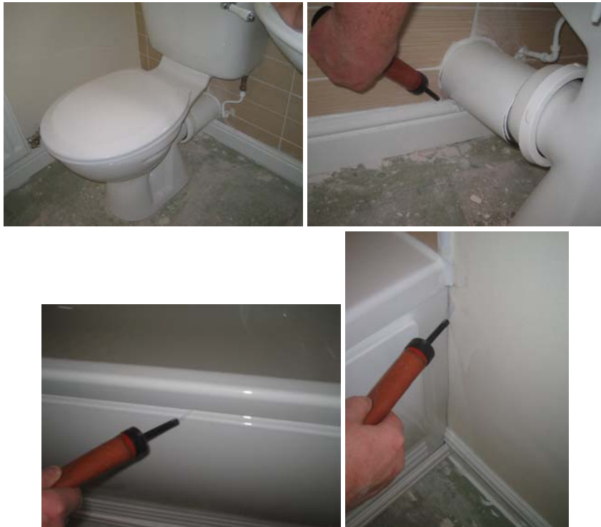
Figure 14.15 Where visible, plumbing penetrations into the service void along the wall in the 1 st floor bathroom were sealed around effectively, in less visible areas the sealing was less successful.
