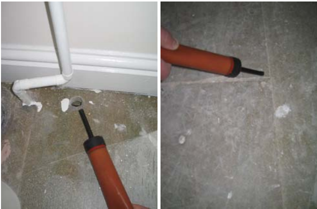
Figure 5.9 Air leakage into the first intermediate floor void through an unsealed hole in the bathroom and gaps between flooring panels in the front bedroom.
