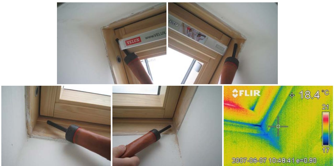
Figure 14.19 All 3 of the rooflights in the 2 nd floor rear bedroom displayed some degree of air leakage.
