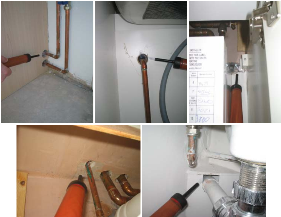
Figure 5.16 Air leakage into voids behind units, plasterboard and ceiling in the kitchen, and into the boxing in the downstairs WC around various plumbing penetrations.
