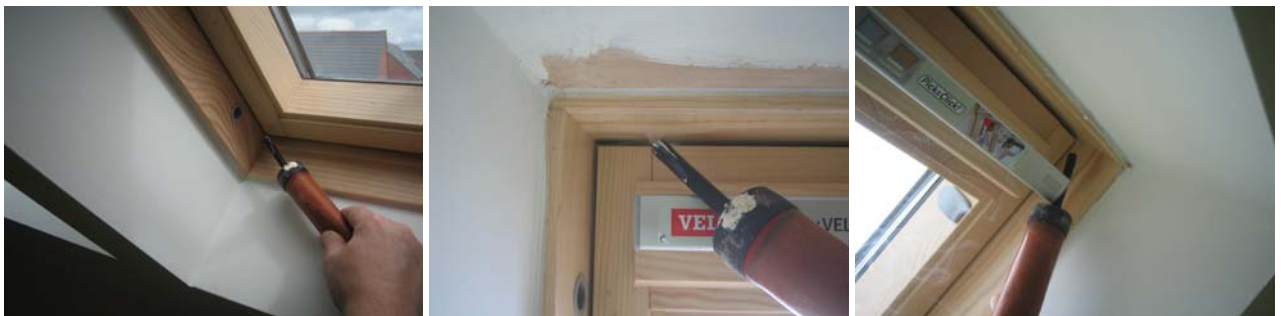
Figure 9.21 All 3 rooflights allowed some direct infiltration.
