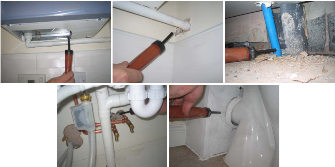
Figure 9.16 Air leakage around ground floor plumbing penetrations in the utility room, kitchen and WC.
