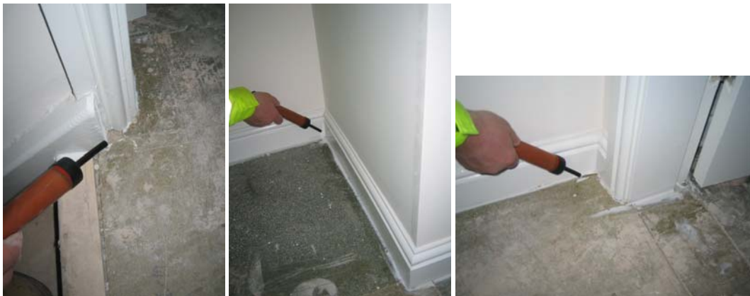
Figure 3.5 Air leakage at the first floor room perimeters in the landing and master bedroom.
