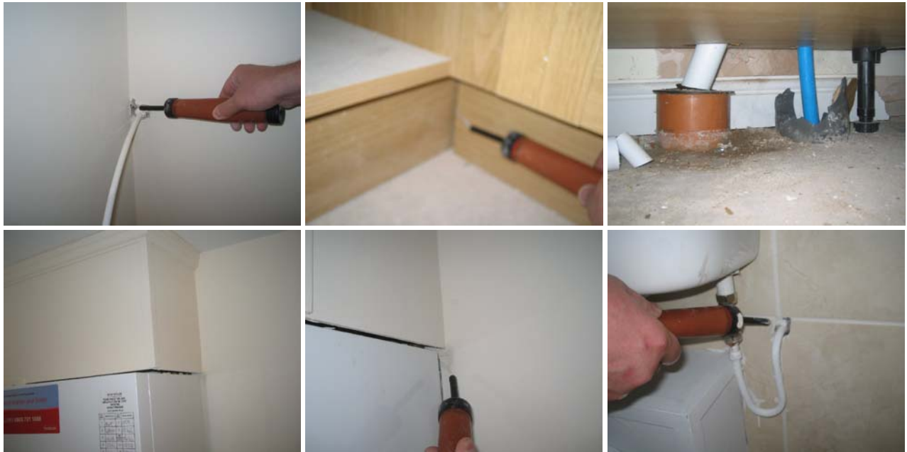
Figure 10.14 On the ground floor around plumbing penetrations in the kitchen (around the water supply for the fridge/freezer and under the units), in the utility room (around the boiler and under the units), and in the downstairs WC.
