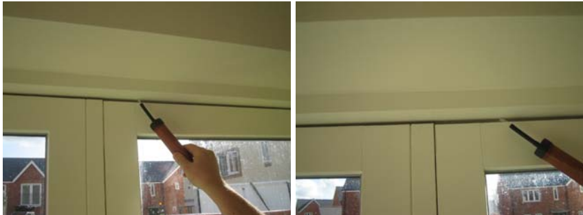
Figure 7.15 Air leakage about an incorrectly set patio door.
