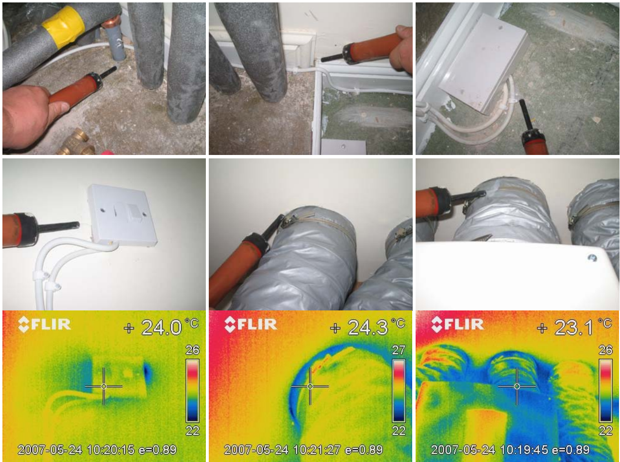
Figure 11.17 Air movement around junctions and penetrations in the 2 nd floor cylinder cupboard.
