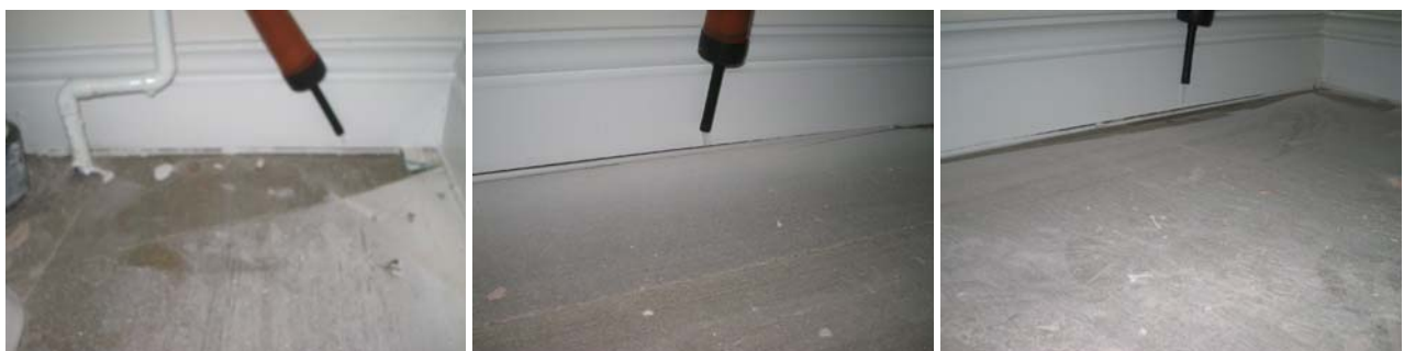
Figure 6.4 Air leakage detected where the sealing of the floor/wall junctions was impaired, either through the presence of debris, insufficient sealant or the sealant had already failed.
