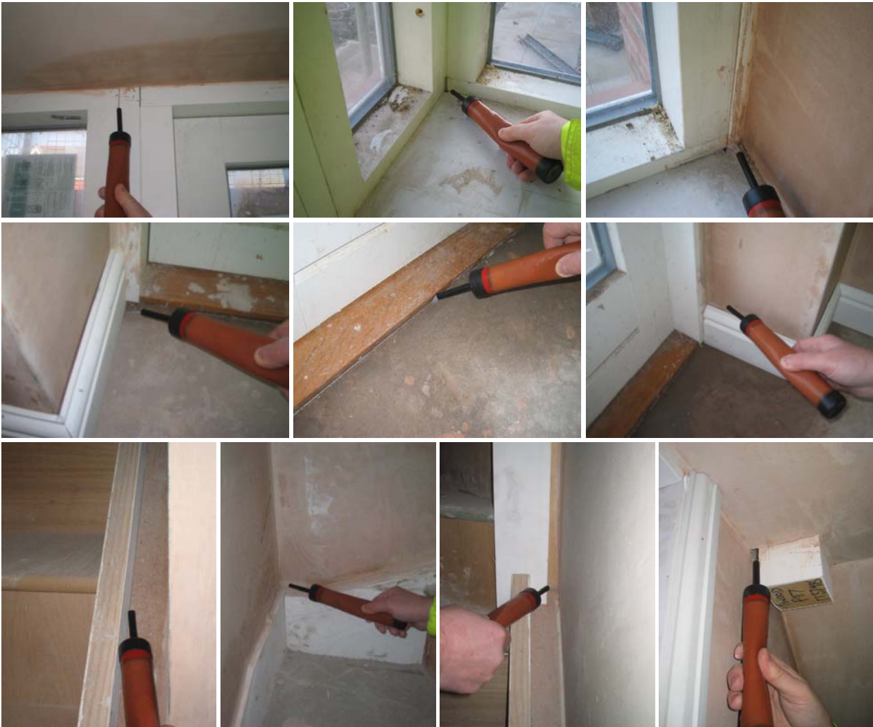
Figure 2.3 Air leakage around the staircase.
