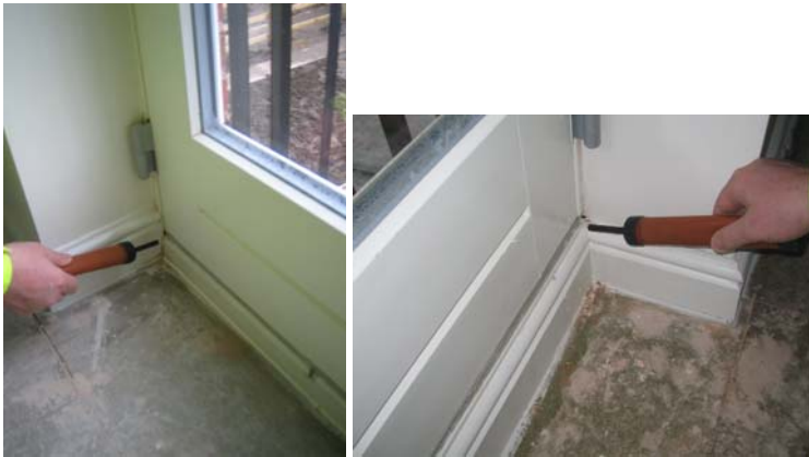
Figure 4.6 Leakage around the patio doors on both the first and second floors.
