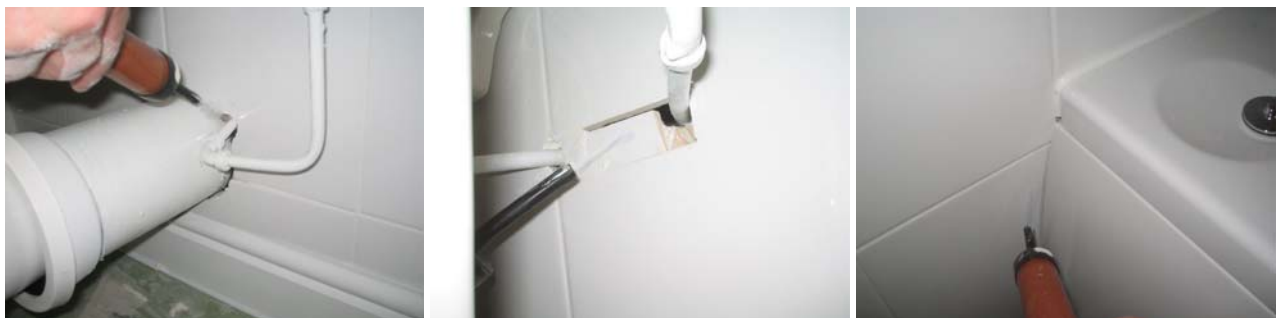
Figure 10.15 Air leakage was detected into the service void in the 1 st floor bathroom around plumbing penetrations for the toilet and basin water supplies and also around the bath panel.
