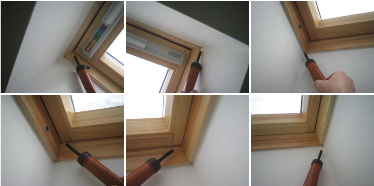
Figure 5.14 Air movement detected around the rooflight casements and frames.
