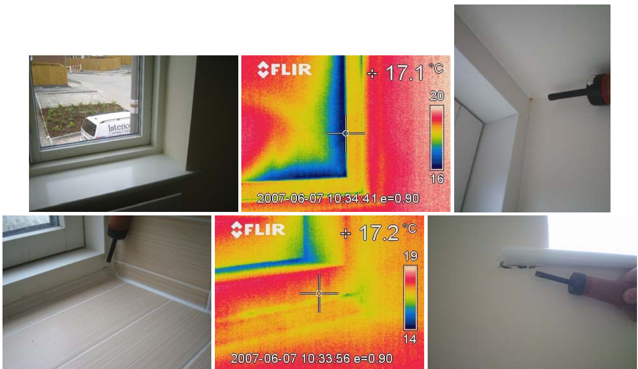
Figure 14.9 The replacement lounge window showing infiltration under depressurisation; and air leakage again detected around the kitchen window frame, the sill in the 1 st floor bathroom and beneath window sills on the 1 st and 2 nd floor even though additional decorating work had been carried out.
