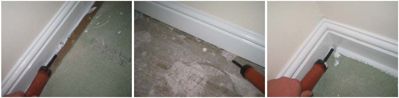
Figure 11.4 Air leakage at the unsealed wall/floor junctions on the 1 st floor; along and internal wall, the separating wall and the corner of 2 external walls.
