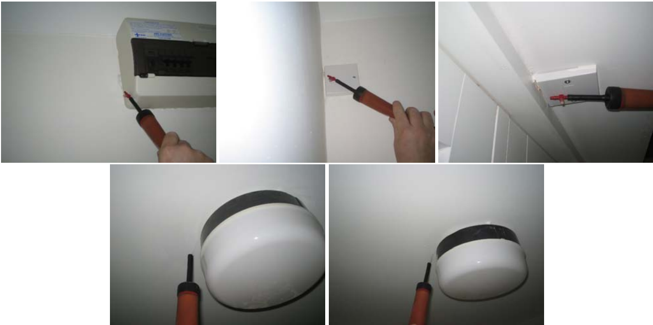
Figure 3.12 Air leakage around electrical penetrations around the consumer unit, electrical fixings in the kitchen and the bathroom/en-suite/WC light fixings
