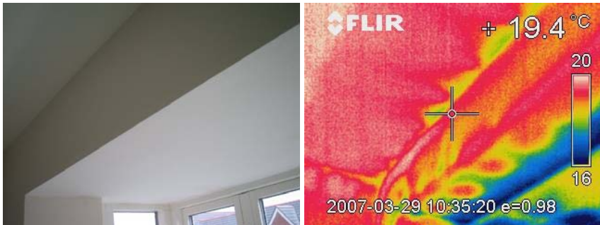
Figure 13.15 A combination of the effects of thermal bridging and air movement at the bay window ceiling.
