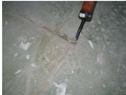
Figure 9.6 Air leakage through a gap in the 2 nd intermediate floor in the front bedroom.
