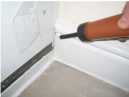
Figure 9.11 Air leakage around the back door threshold.
