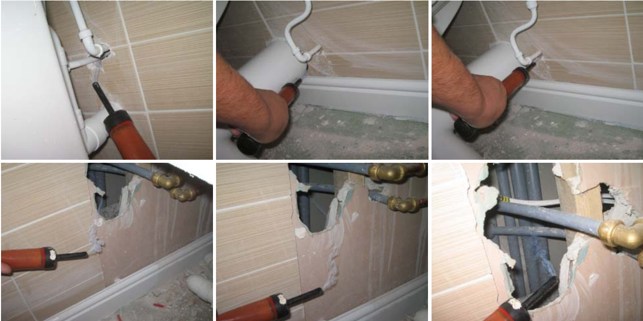
Figure 11.15 Air movement around unsealed plumbing penetrations in the 1 st floor bathroom.
