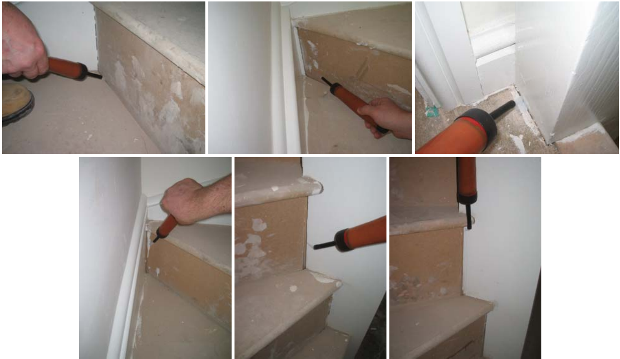
Figure 7.16 Air leakage into the voids surrounding both sets of stairs.
