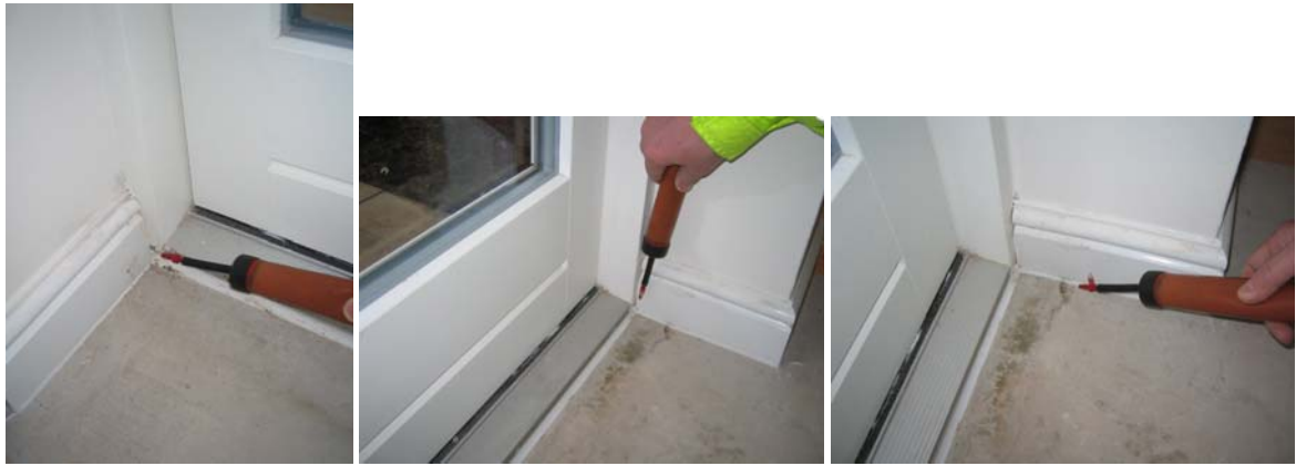
Figure 3.3 Air movement around the patio door threshold in the kitchen.
