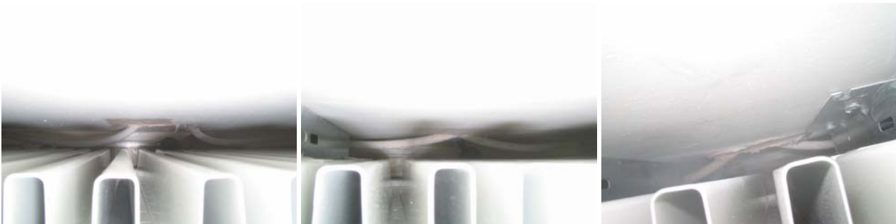
Figure 5.15 Leakage behind the radiators on the first and second floors.
