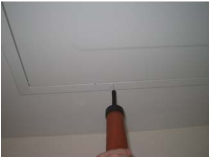
Figure 5.13 Leakage between the loft trap and door.
