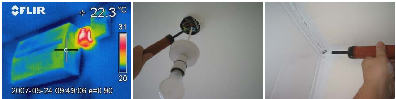
Figure 11.11 Around electrical penetrations on the ground floor a small amount of air movement was detected behind the consumer unit, through central light fixings and around wiring for the security system.
