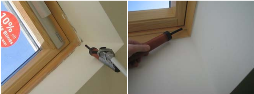
Figure 7.25 Air leakage at the rooflights in both the kitchen/diner and in the second floor rear bedroom.
