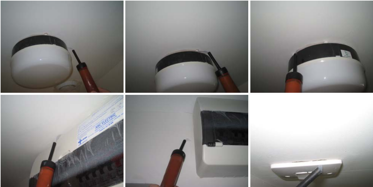
Figure 5.17 Air movement around the bathroom, en-suite and downstairs WC light fixings, around and through the electrical consumer unit and around an electrical penetration on a second floor internal wall.
