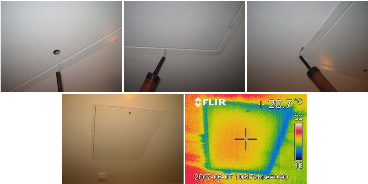
Figure 14.20 Infiltration at the loft hatch was again detected through the loft hatch keyhole, between the hatch and door, and around the frame itself.
