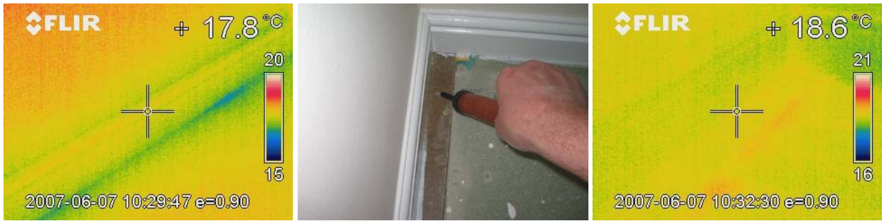
Figure 14.5 Under depressurisation, cooler air entering at the 1 st floor on external walls, whereas on internal walls there was no temperature difference with warmer air emerging from gaps between flooring panels.
