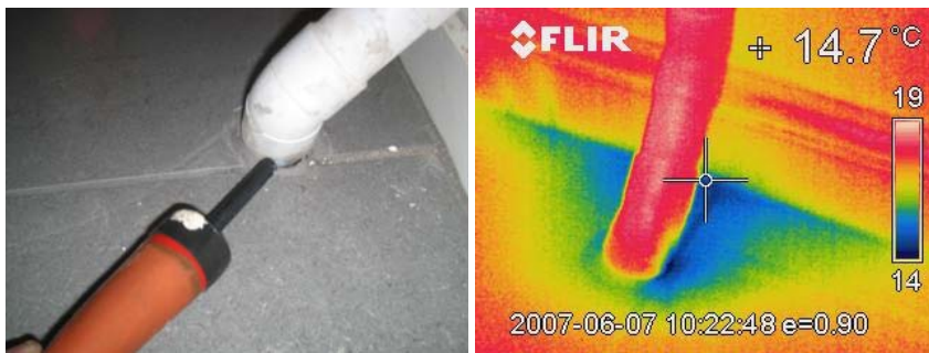
Figure 14.14 Air leakage around the waste pipe for the basin in the ground floor WC.
