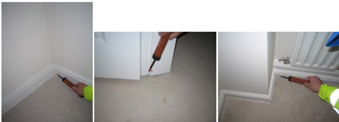
Figure 3.2 Leakage at the ground floor perimeter in the kitchen and utility room.
