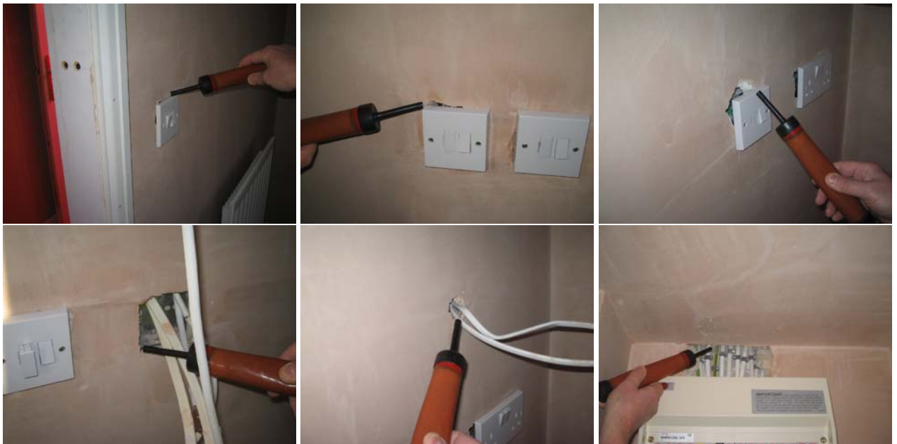
Figure 1.6 Ground floor electrical service penetrations.
