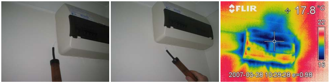
Figure 12.13 Air leakage around the electrical consumer unit.
