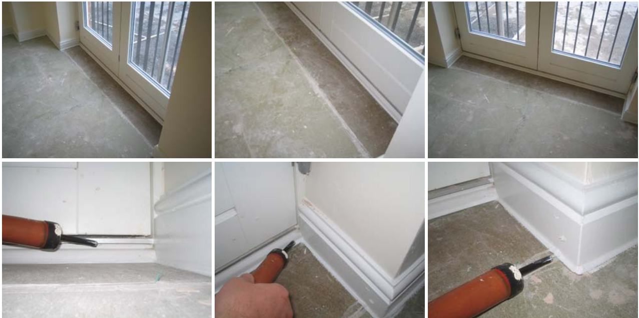
Figure 10.10 The 1 st floor balcony doors had been sealed well, with only a small amount of air leakage detected at the threshold and around the skirting board at the return.
