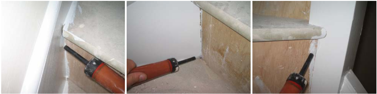
Figure 11.10 Air movement through gaps in the staircase between the 1 st and 2 nd floors.
