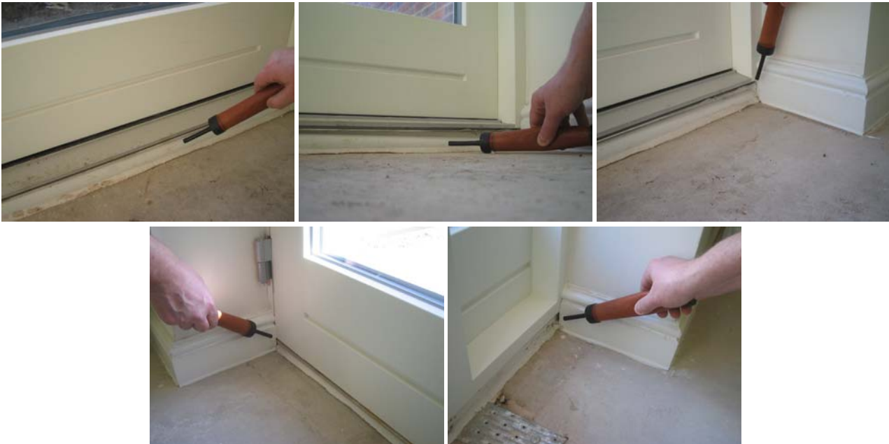
Figure 7.13 Air leakage through gaps around the patio door and rear door thresholds in the kitchen.
