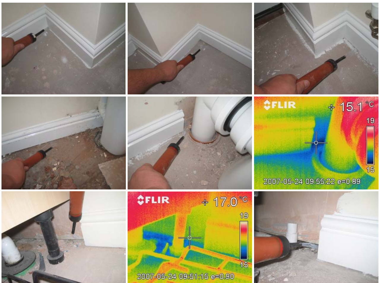
Figure 11.3 Air leakage at wall/floor junctions on the ground floor, under the skirting in the dining room and utility room, in the downstairs WC, and in hidden areas behind units in the kitchen and utility.
