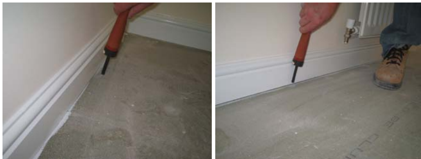
Figure 14.6 Infiltration detected at wall/floor junctions in the 2 nd floor front and rear bedrooms on the party and external walls.
