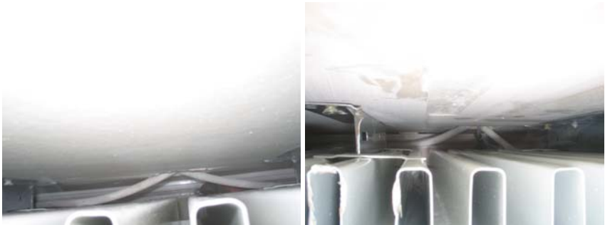
Figure 10.18 Behind the radiators air movement into the walls, around the pipework, was normal, examples shown are from the a first floor bedroom on an external wall and from the ground floor WC on a masonry internal wall.
