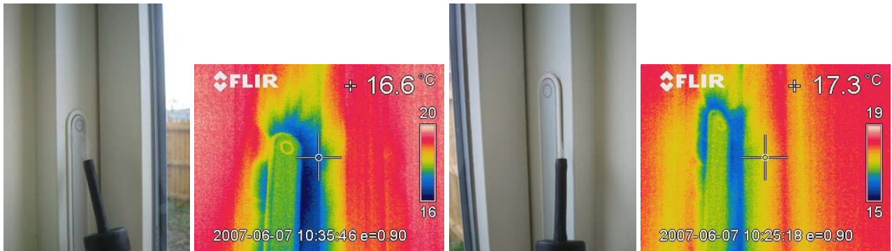
Figure 14.10 Air leakage at the trickle vents in the kitchen window.
