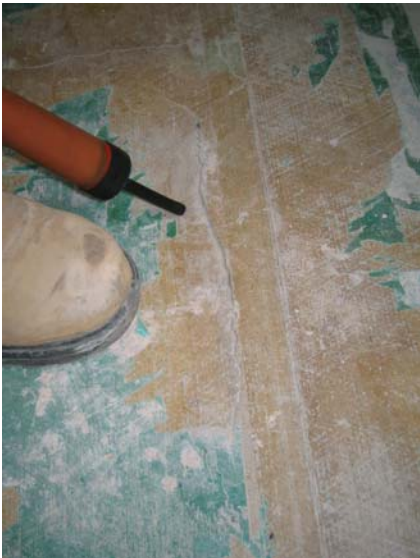
Figure 8.9 Damage to the intermediate floor in the front bedroom.
