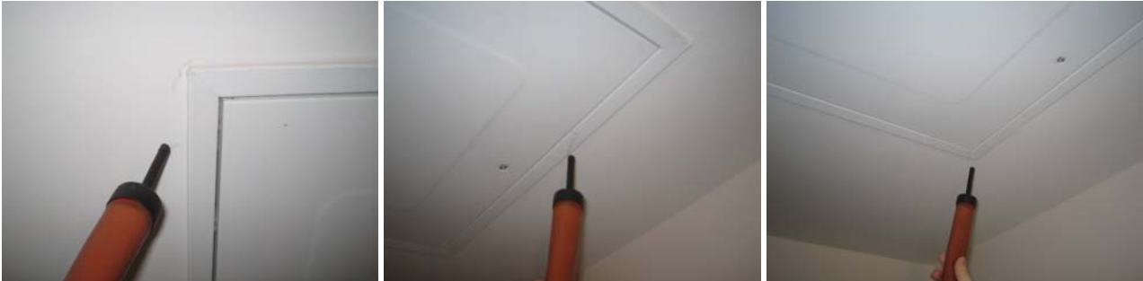
Figure 3.10 Direct air leakage around the loft hatch.
