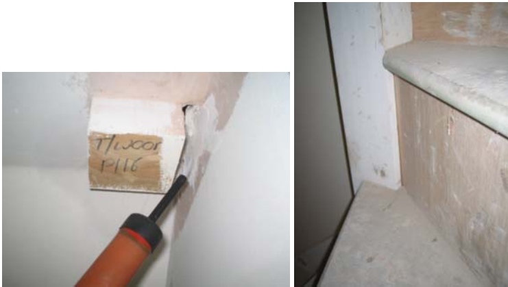
Figure 8.5 Gaps around the stairs remaining unsealed.
