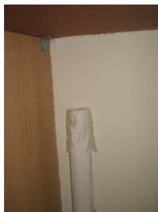
Figure 7.2 Temporary sealing to the washing machine waste pipe.
