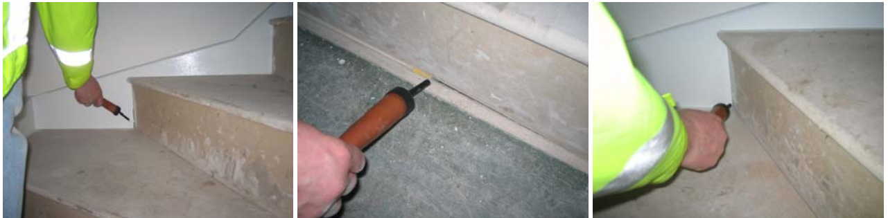
Figure 3.4 Air leakage detected around steps and risers of both staircases.
