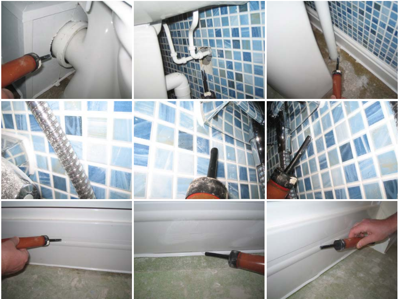
Figure 9.18 Air leakage around 2 nd floor plumbing penetrations in both en-suite bathrooms, with no sealant applied to the underside of the shower control unit. Air leakage around the shower tray fascia panels was far less than expected due to capably applied sealant.
