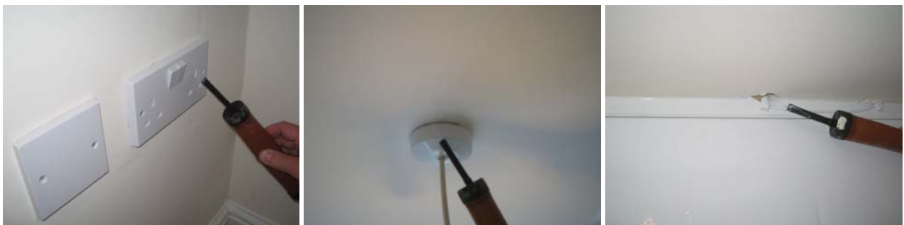
Figure 10.11 Air leakage around ground floor electrical penetrations in the dining room, kitchen and utility room.
