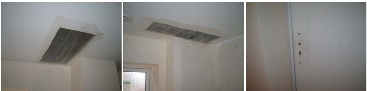
Figure 11.2 Temporary sealing in the kitchen, 1 st floor bathroom and over penetrations through the back door in the utility room.
