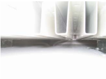
Figure 7.20 Leakage through the pipework penetrations for the radiator in the first floor bathroom.
