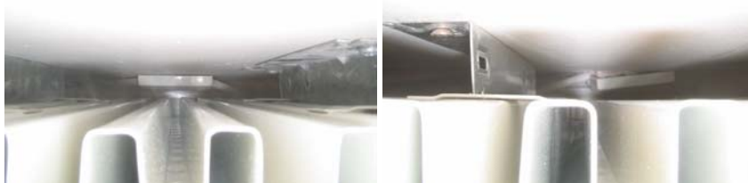
Figure 11.18 Leakage was detected around the radiator pipework behind the radiators, which appeared most severe on internal partition walls.
