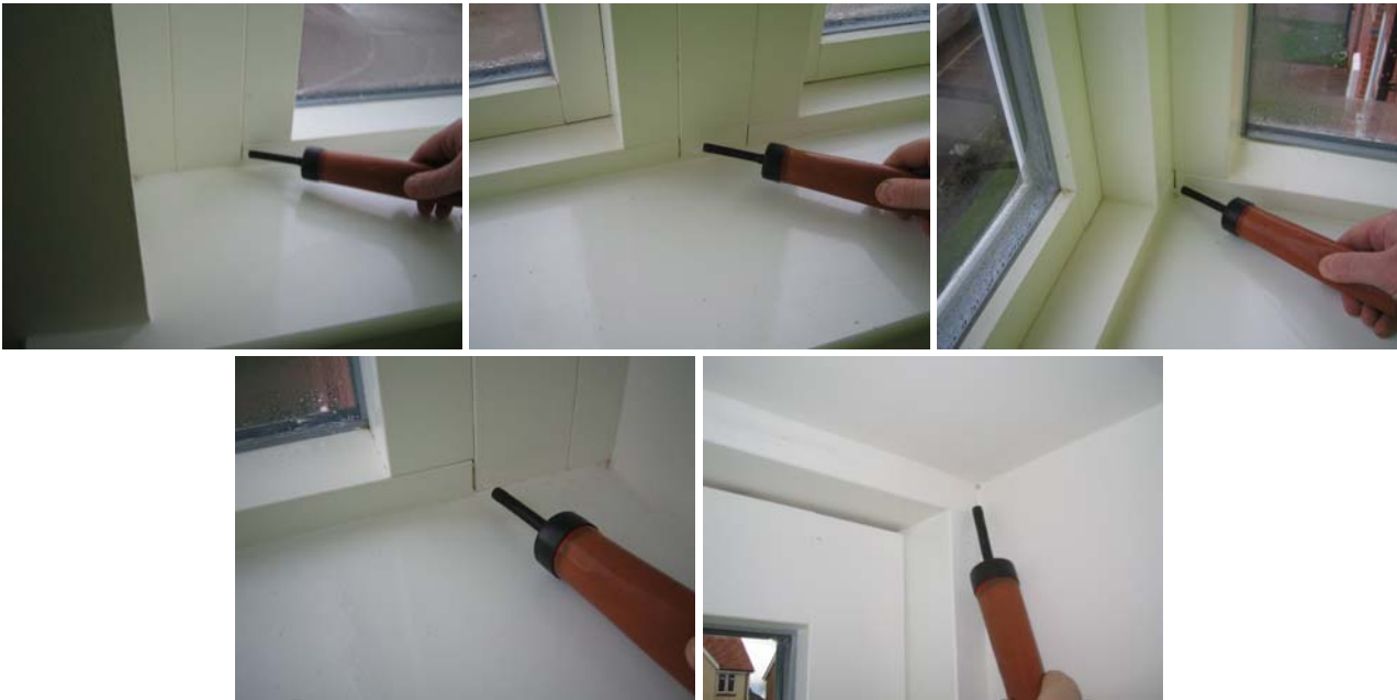
Figure 4.10 Leakage detected between elements of the first floor bay window and around the frame of the patio door in the kitchen.
