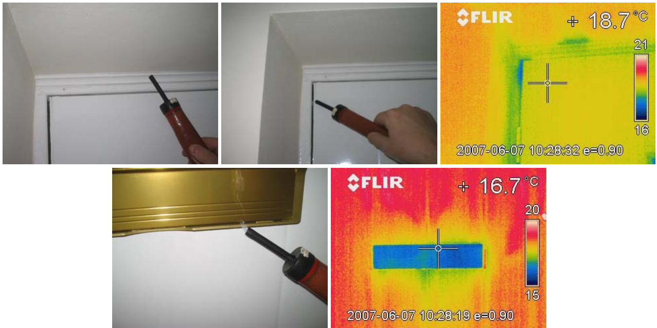
Figure 14.8 Air leakage at the head of the front door, around the door casement on the hinge side and around the letterbox.
