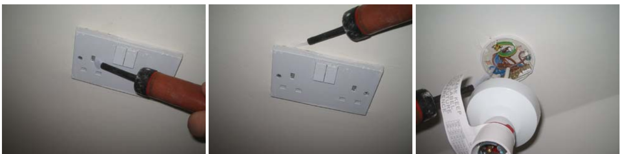
Figure 11.13 Indirect air leakage into walls and direct leakage into the loft space around electrical penetrations on the 2 nd floor,
