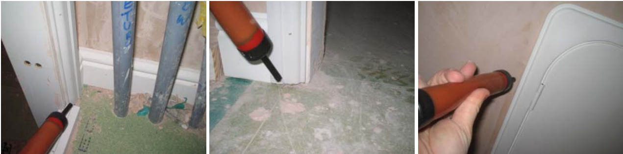
Figure 2.10 Air movement through unsealed junctions on the first floor
