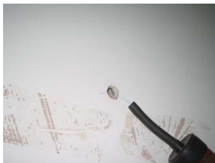
Figure 12.2 Air leakage into the void behind the plasterboard on the party wall, under dwelling pressurisation, through a hole drilled for placement of the thermocouples during the coheating test.
