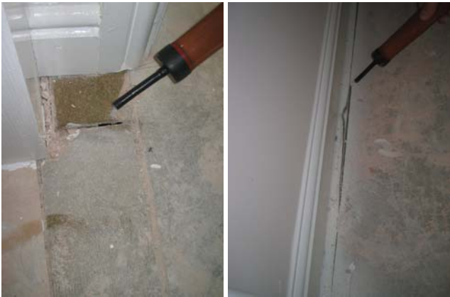
Figure 5.11 Movement of air through gaps in the second intermediate floor on the landing and in the rear bedroom cupboard.
