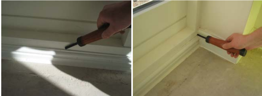
Figure 7.14 Leakage around the frame of the kitchen gallery window.
