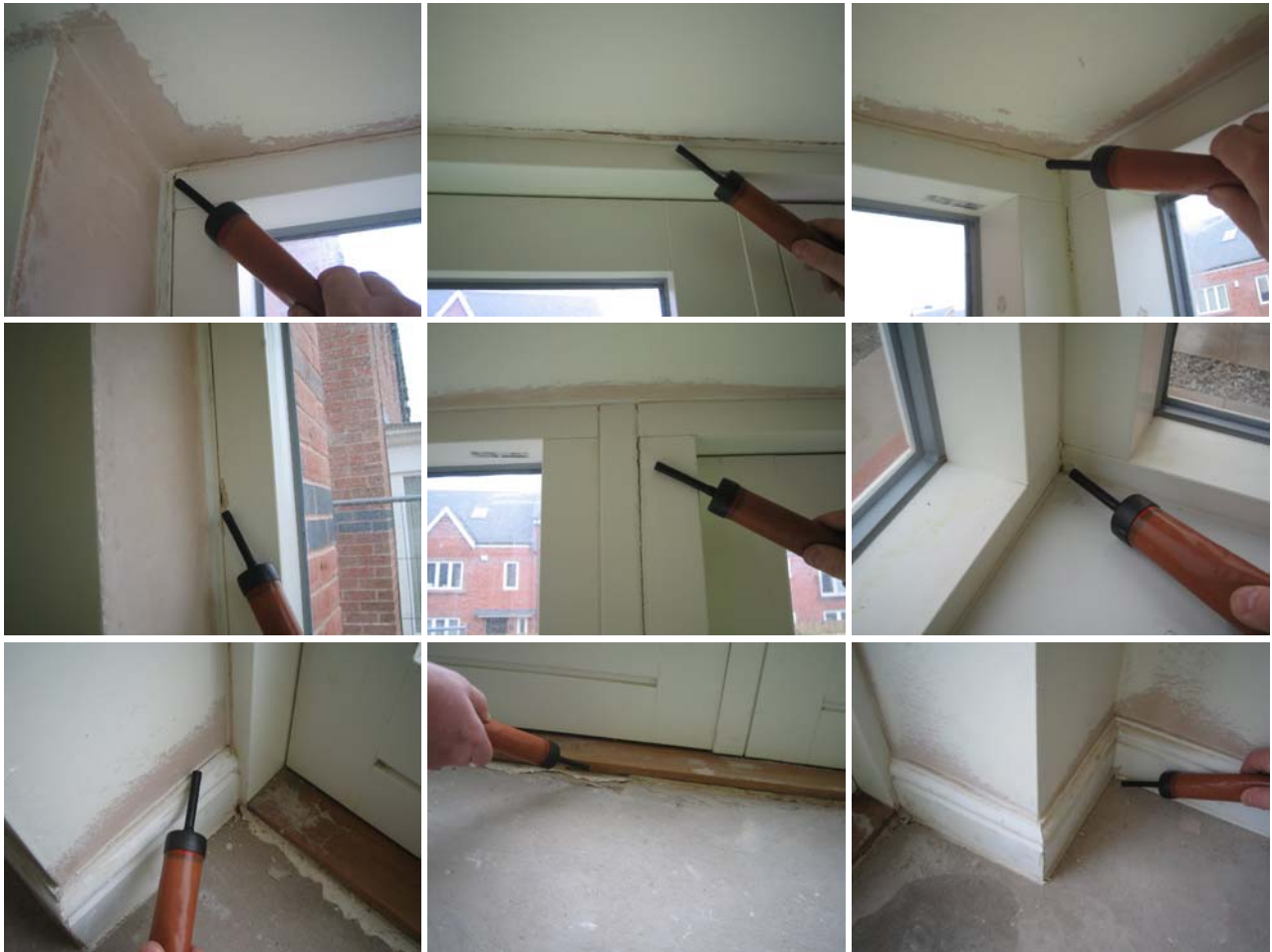
Figure 8.3 Air leakage at various places around the ground floor bay window.
