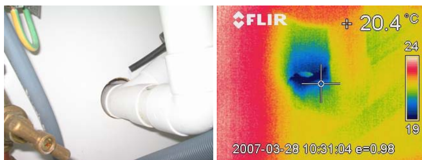
Figure 12.12 Air movement around the penetration for the kitchen sink waste pipe.
