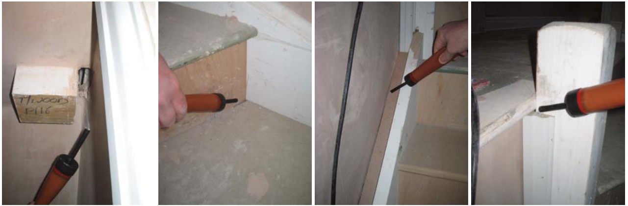
Figure 1.5 Air leakage around the staircase.
