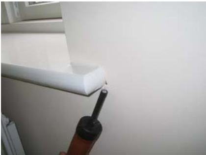
Figure 9.12 Very little air movement was detected around the windows, this small hole at the sill in the dining room was one of the few examples observed.
