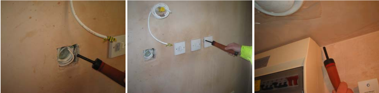
Figure 2.4 Ground floor electrical penetrations.
