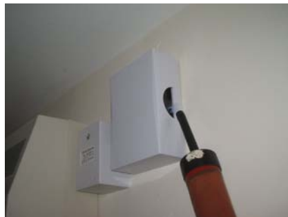
Figure 14.12 Movement of air through electrical penetrations on the ground and 1 st floor electrical penetrations was the same as that observed in the initial test.
