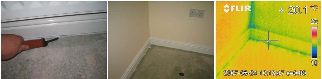
Figure 11.6 Infiltration detected at wall/floor junctions in the 2 nd floor front bedroom on the external wall and adjacent party wall.
