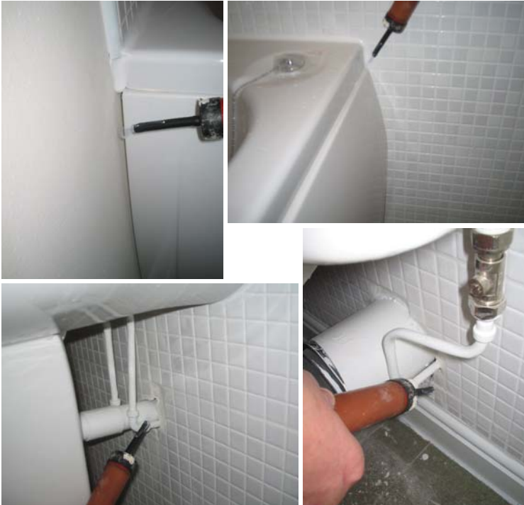
Figure 9.17 Air movement in the 1 st floor bathroom was detected into the void under the bath and around plumbing penetrations into the service void.
