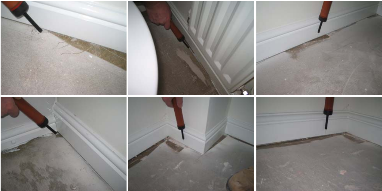
Figure 5.8 Leakage was observed at almost all points around the first floor perimeter, on internal, separating and external walls.
