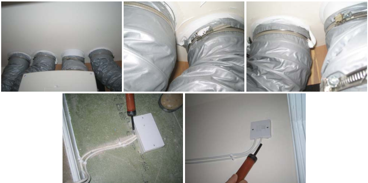
Figure 10.17 In the cylinder cupboard air leakage directly into the loft around the ventilation ducting was reduced from that observed in plot B119, but still detectable. Air movement through electrical penetrations in both the floor and wall was appreciably larger than in plot B119.
