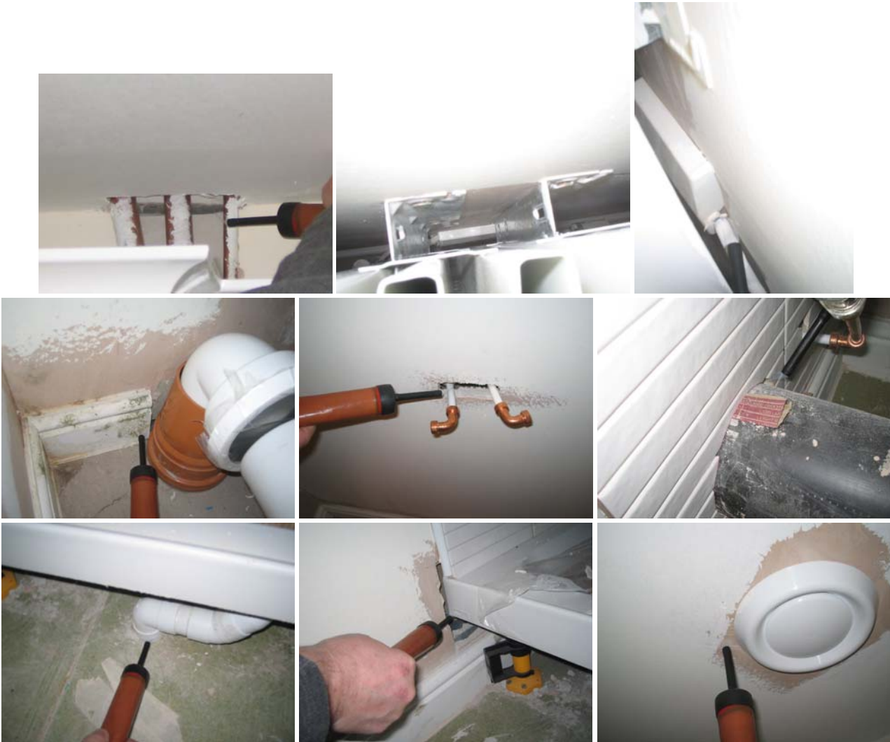
Figure 8.7 Air leakage around various penetrations for heating, plumbing and ventilation services.
