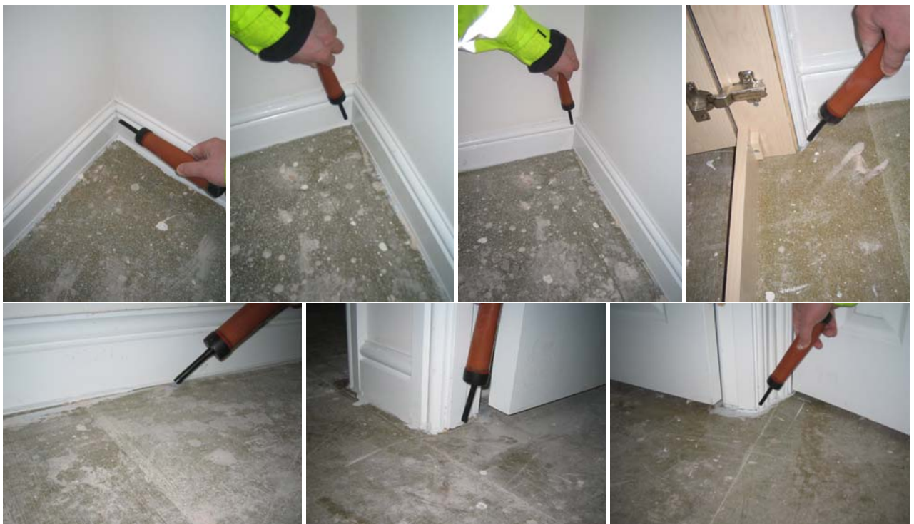
Figure 3.8 Air leakage around the wall/floor junctions on the second floor.
