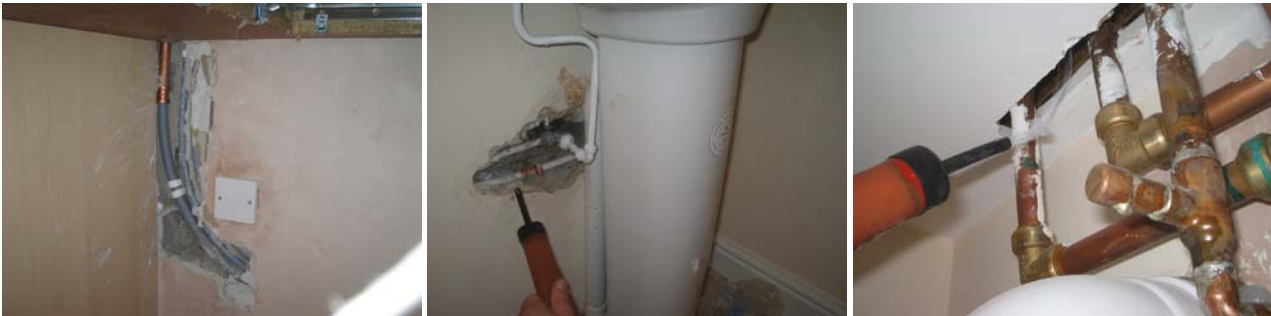
Figure 11.14 Unfinished plumbing penetrations on the ground floor.
