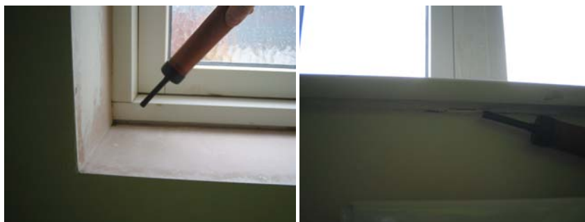
Figure 8.4 Air leakage at window sills.
