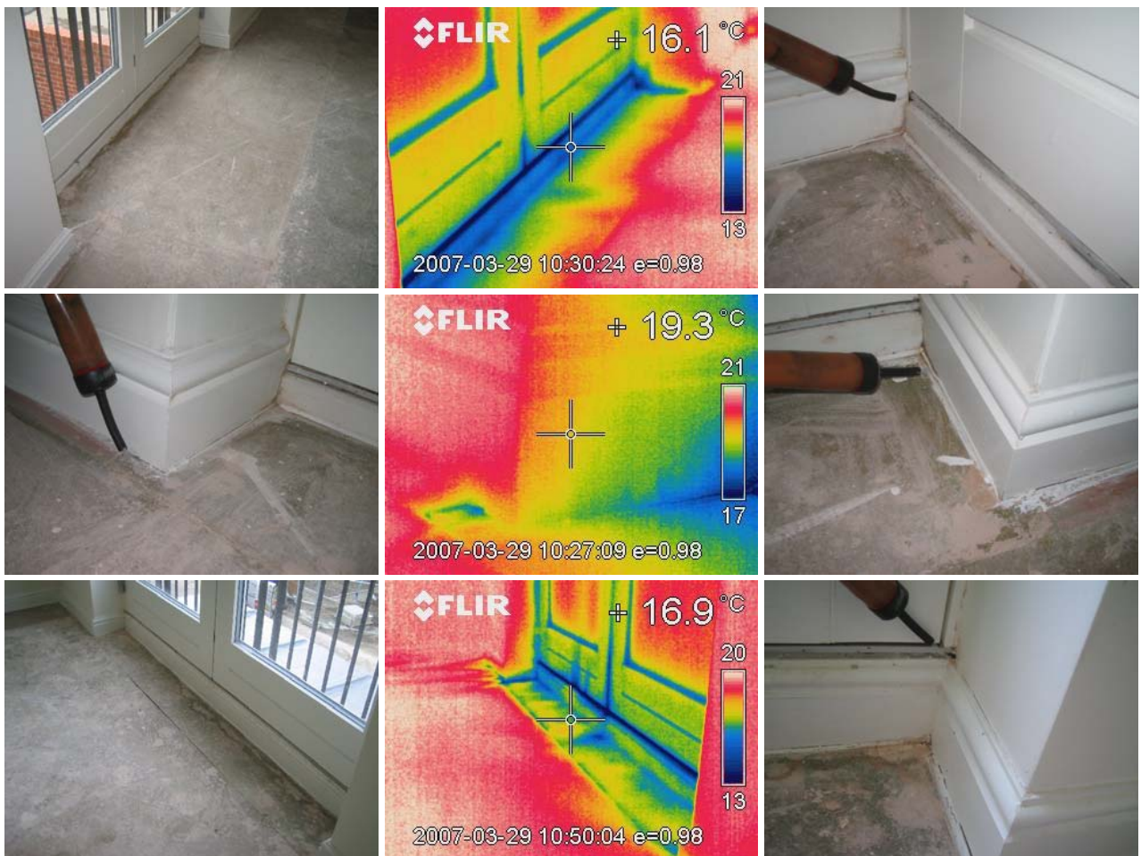
Figure 13.6 Air leakage around the bottoms of the balcony doors on the 1 st and 2 nd floors
