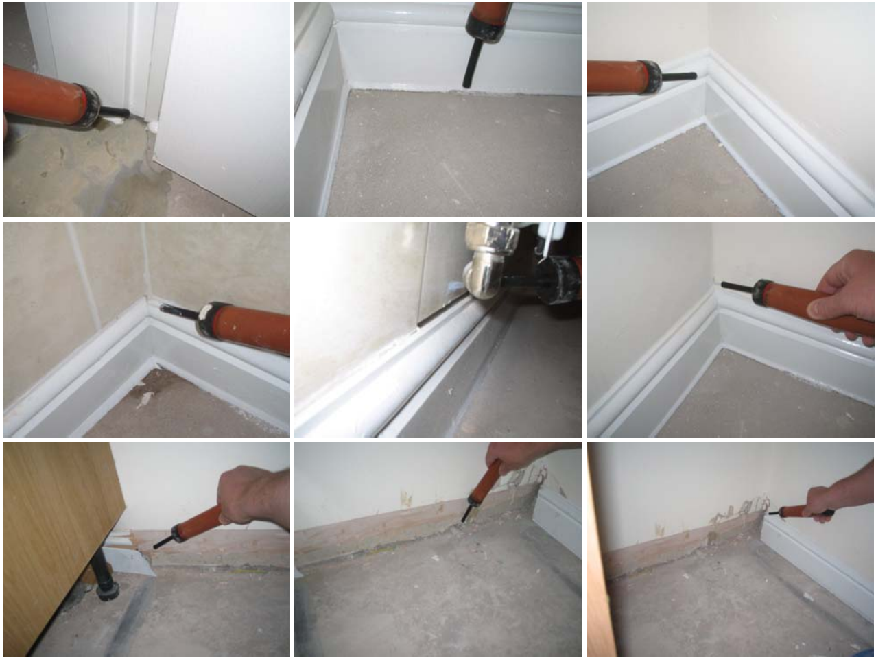
Figure 10.3 Air leakage at a doorframe and under the skirting in the dining room, and at junctions and over the skirting in the kitchen, WC and dining room. More significant leakage at the unfinished floor/wall junction in the utility room.
