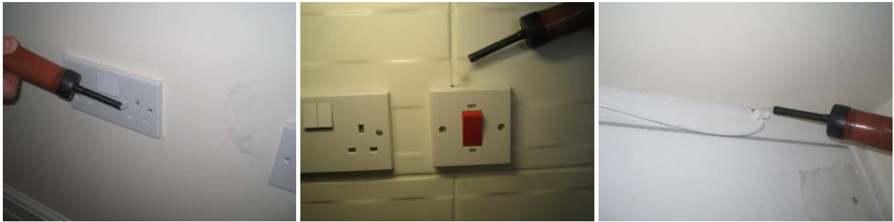
Figure 9.13 Air leakage through ground floor electrical penetrations in the dining room, kitchen and utility room.
