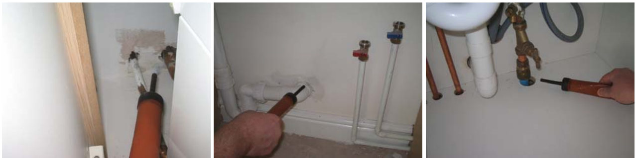
Figure 7.22 Gaps around plumbing penetrations in the kitchen allowing air leakage into intermediate floor void, the void behind the plasterboard and the void behind the kitchen units.
