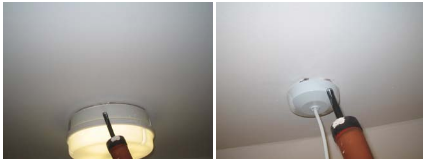
Figure 10.13 Direct air leakage into the loft space around light fittings in an en-suite and the rear bedroom.
