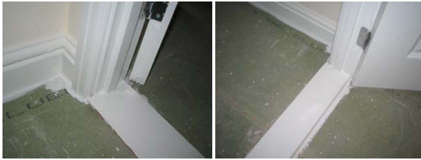
Figure 10.6 No air leakage was detected around the floor perimeters in the 2 nd floor bedrooms due to the well applied sealant, even in the less visible areas such as the built-in wardrobe.
