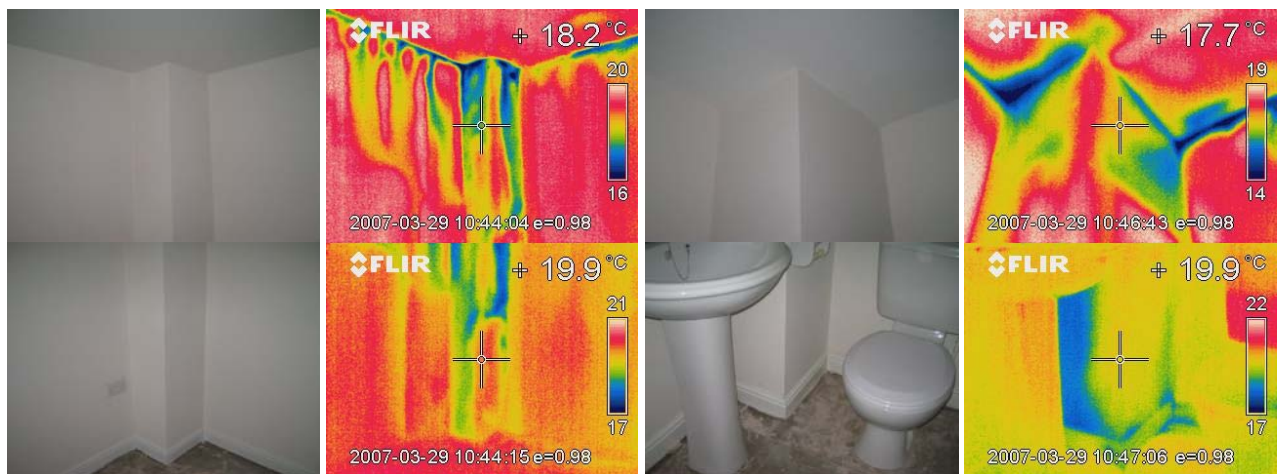
Figure 13.17 Air leakage into 2 nd floor service voids in both bedroom and bathroom.
