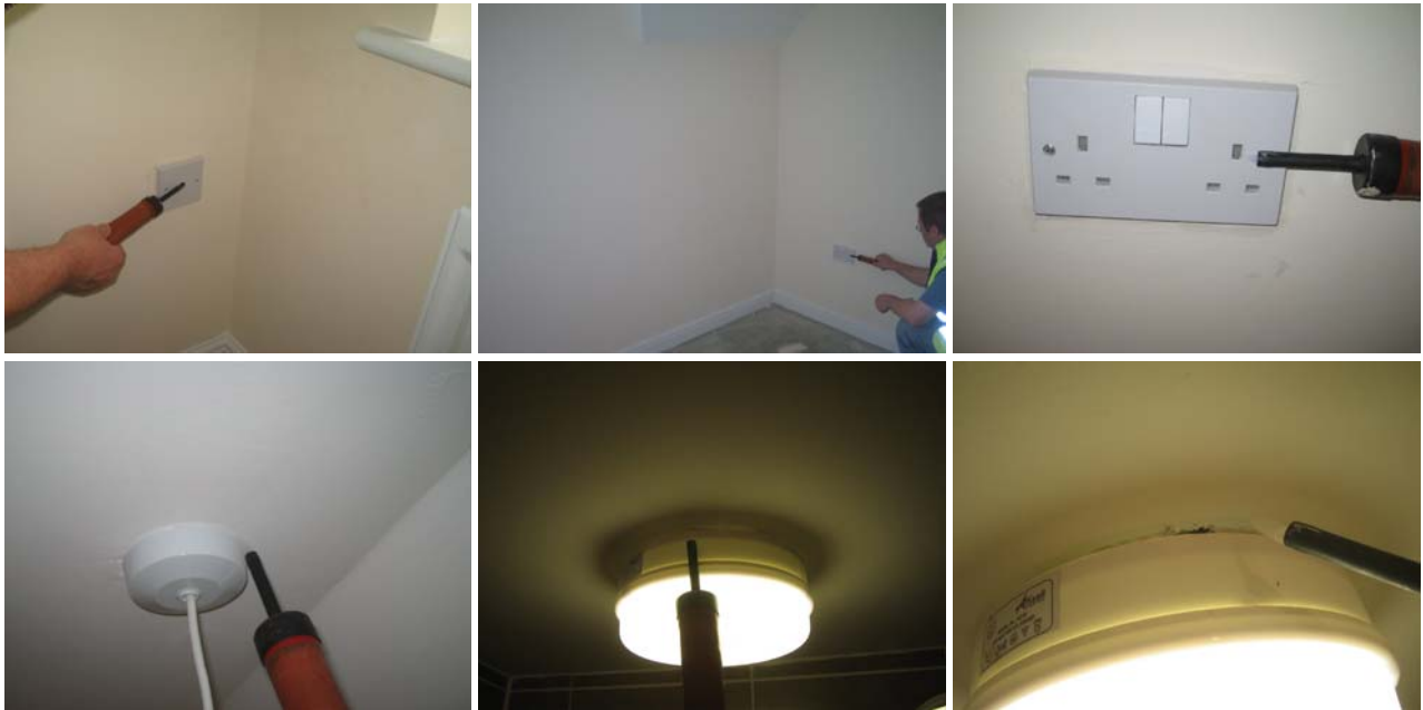
Figure 14.13 Indirect air leakage into walls and direct leakage into the loft space around electrical penetrations on the 2 nd floor,
