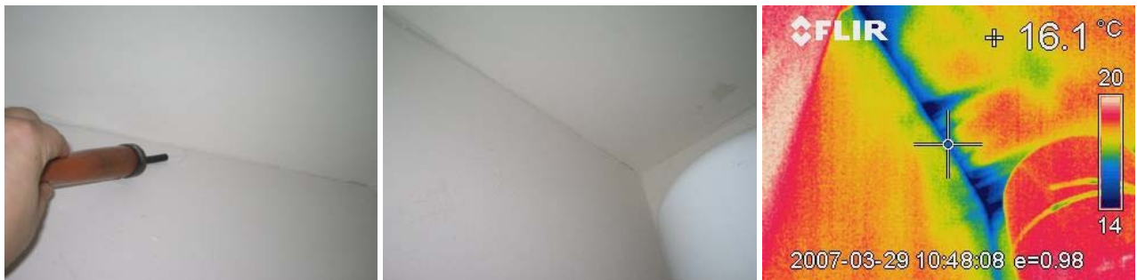
Figure 13.9 Air leakage at the cylinder cupboard ceiling.
