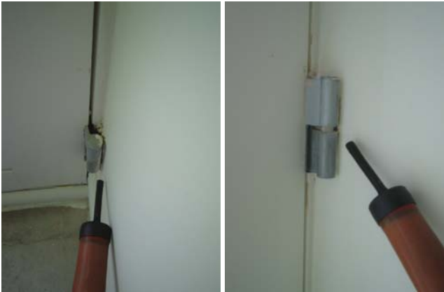
Figure 5.6 Air leakage around external door hinges in the kitchen.
