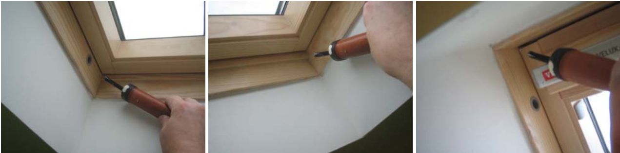
Figure 10.19 Air leakage through the rooflights in the 2 nd floor rear bedroom.
