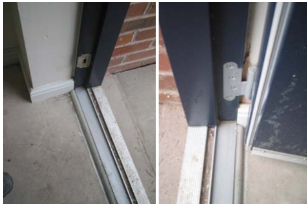
Figure 5.3 Gaps around the front entrance which were inaccessible during the test.
