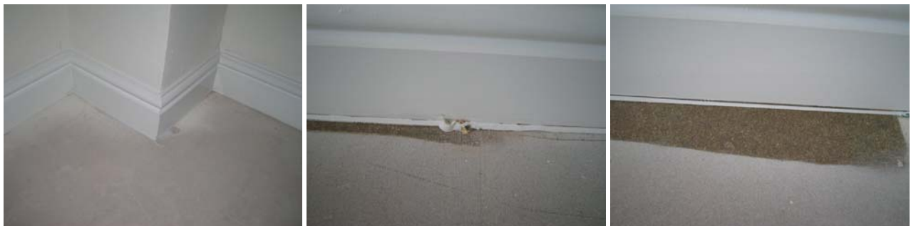
Figure 6.3 Examples of floor/wall junctions; well-sealed, with debris beneath the sealant, and failed joints.
