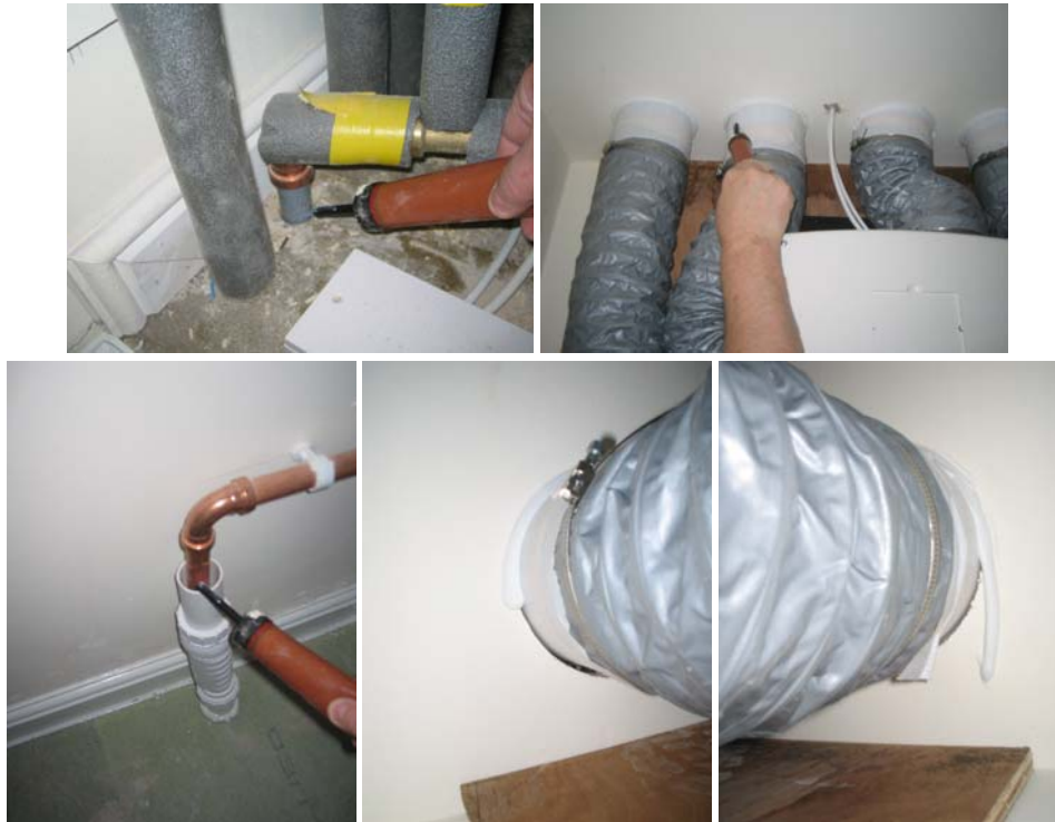
Figure 9.19 Air leakage around penetrations into the cylinder cupboard floor and ceiling, and photographs showing where the sealant was not applied comprehensively.
