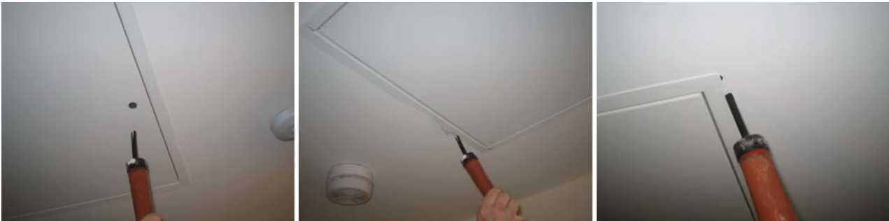
Figure 9.22 Air movement directly into the roof space through and around the loft hatch.
