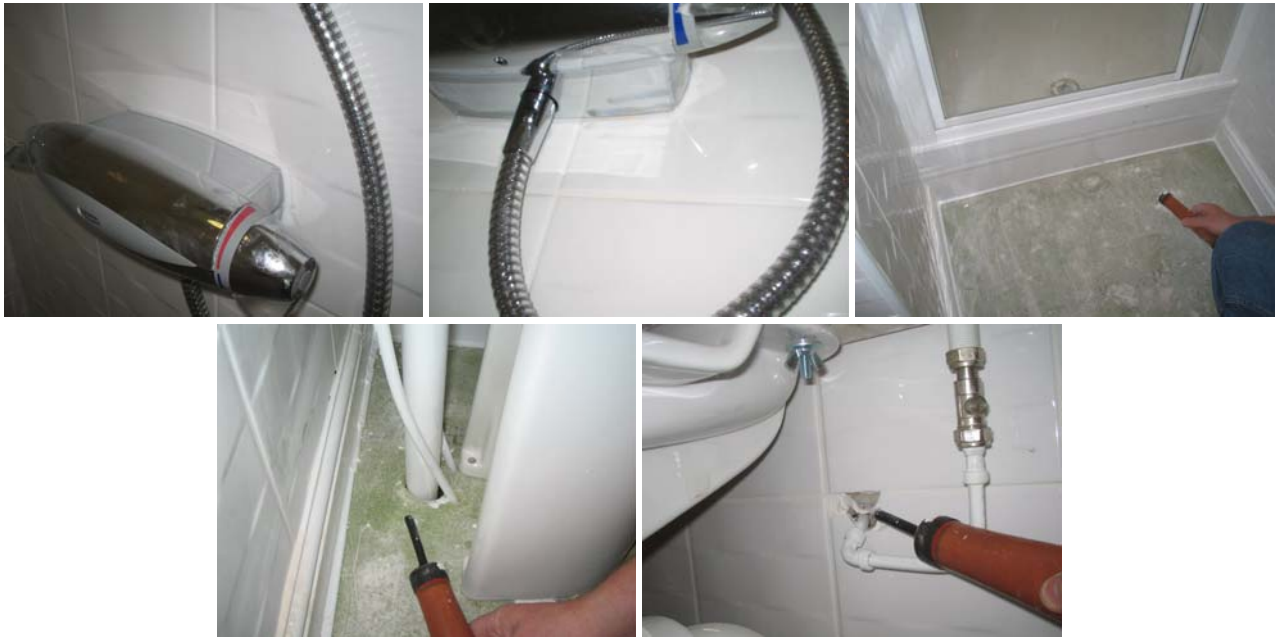
Figure 10.16 On the 2 nd floor the en-suite off the front bedroom had all plumbing penetrations sealed around very well except the shower control unit and air leakage was also detected between the shower tray and fascia panel; in the en-suite off the rear bedroom air leakage was observed around most floor and wall penetrations as they had not yet been sealed.
