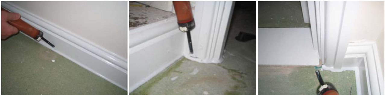
Figure 9.7 The 2 nd floor/wall junctions performed very well apart from a few small gaps around the rear bedroom perimeter and in less visible areas, such as inside the cylinder cupboard and front bedroom built-in wardrobe.
