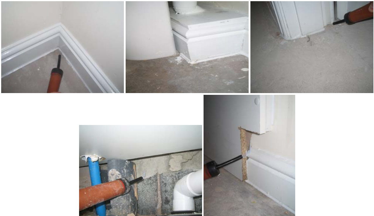
Figure 9.4 Minor air leakages at gaps in the sealant on the ground floor perimeter and at unfinished junctions in the utility room.
