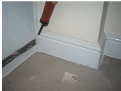
Figure 10.8 At the rear door threshold leakage was detected only at the frame/skirting board junction.
