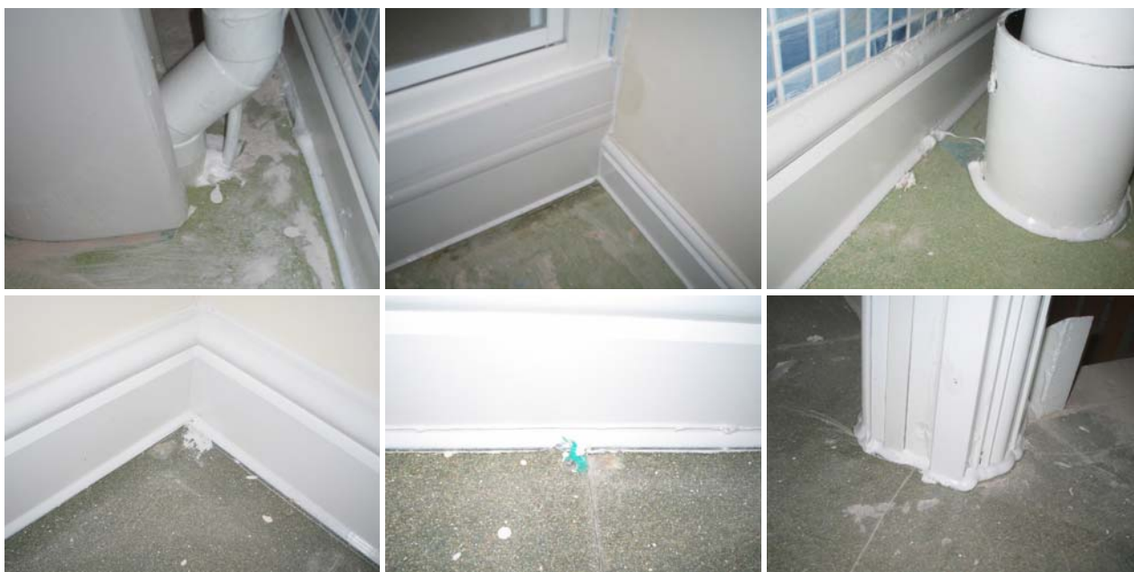
Figure 9.3 A high standard of secondary sealing of many service penetrations and wall/floor junctions was observed throughout most of plot B119.
