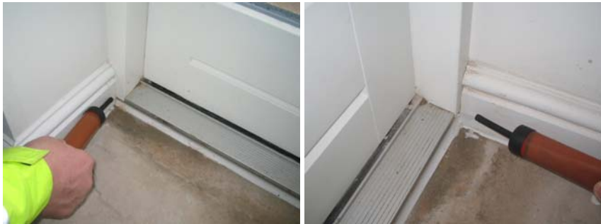
Figure 4.3 Leakage through gaps around the patio door threshold in the kitchen.
