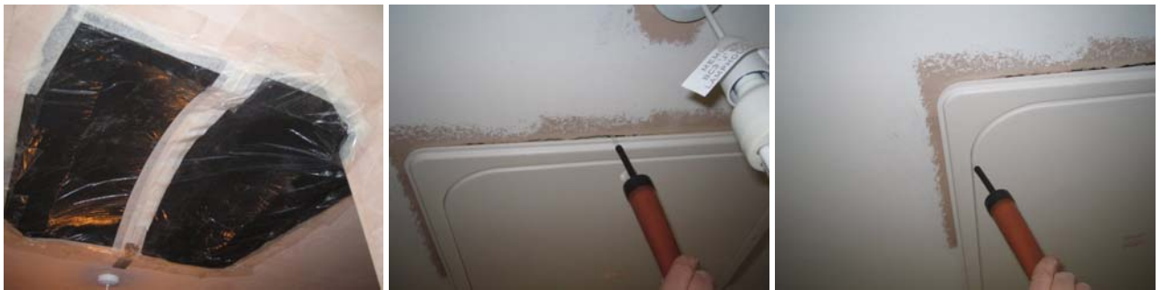
Figure 8.12 The temporary sealing of the loft hatch when the dwelling was previously tested compared with leakage around and through the loft hatch observed during the re-test.
