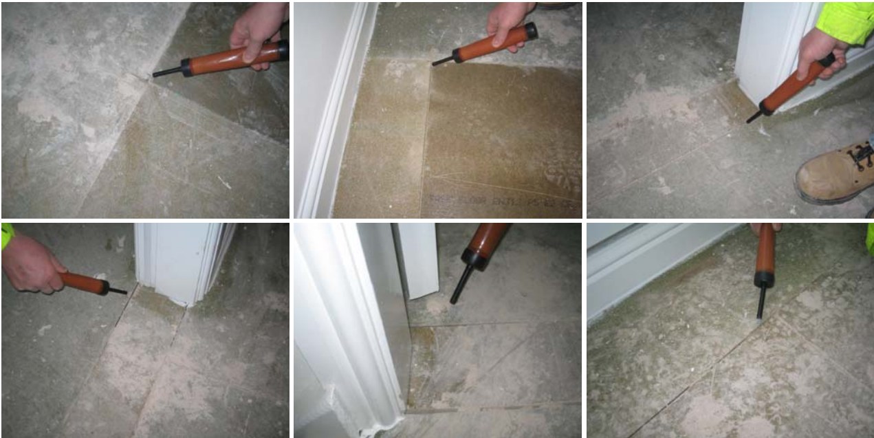
Figure 4.7 As in R110 leakage was observed into both intermediate floor voids through gaps between flooring panels, again this appeared most severe just in front of the patio doors.
