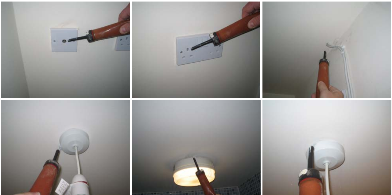
Figure 9.15 Air movement through 2 nd floor electrical sockets in the front bedroom, and into the loft via cables in the cylinder cupboard and light fixings in the landing, en-suite and rear bedroom.
