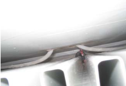
Figure 3.11 Air movement around the radiator pipework.
