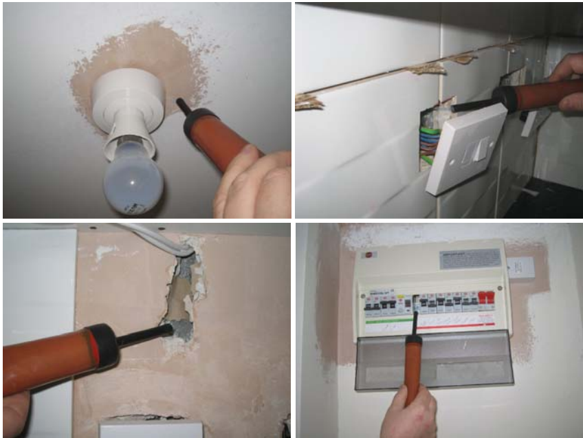
Figure 8.6 Detected air movement at electrical service penetrations:
