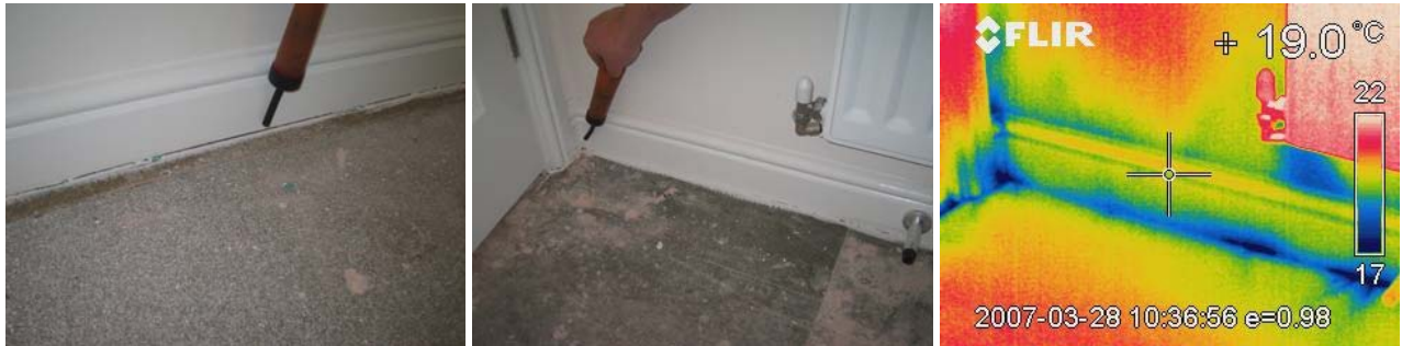
Figure 12.6 Air movement through gaps at the 1 st floor junction with separating and external walls.
