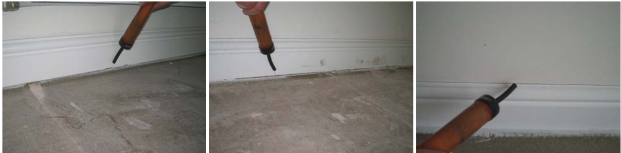
Figure 13.8 Air leakage at the 2 nd floor/wall junctions.
