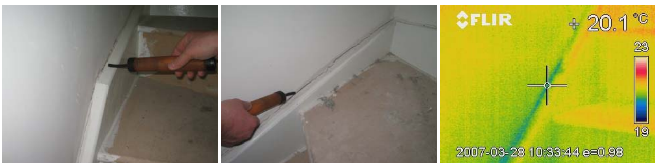
Figure 12.4 Air leakage around the stairs.
