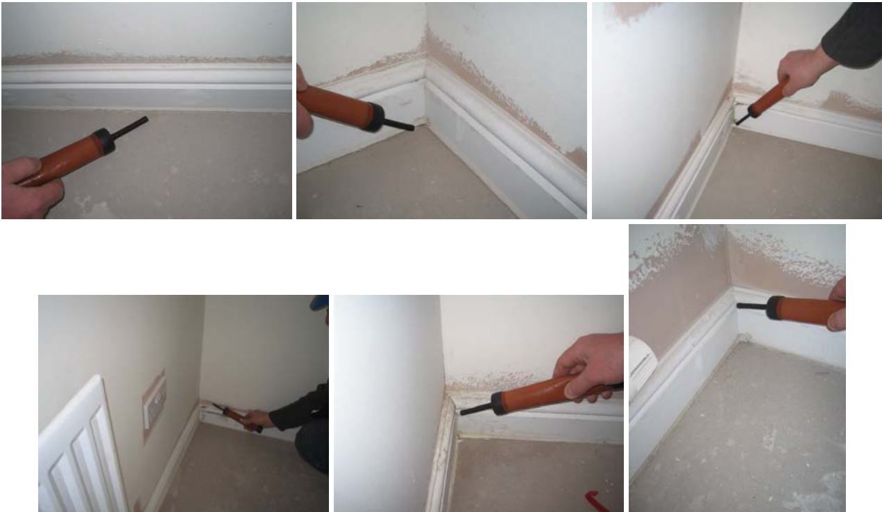
Figure 8.10 Junctions of the ground floor with external and separating walls displayed points of air leakage, this was particularly noticeable at room corners.
