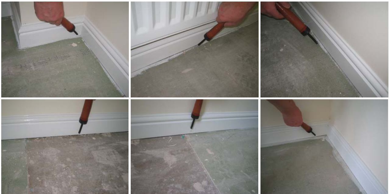
Figure 14.4 Air leakage at the unsealed wall/floor junctions on the 1 st floor; detected along all external and separating walls.
