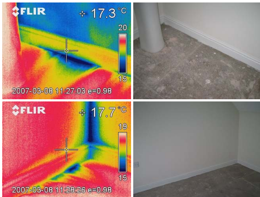
Figure 7.6 Air leakage at the second floor perimeter; at an external wall in the bathroom and at the junction of the separating and wall in front of a warm sloping roof void in the rear bedroom.
