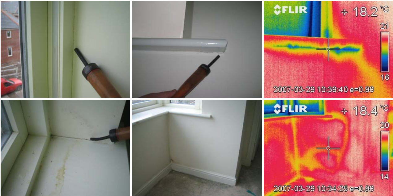
Figure 13.14 Air movement through gaps around the window frame and sills.
