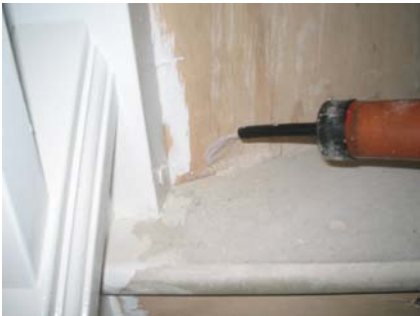
Figure 9.9 leakage at the stairs between the 1 st and 2 nd floors
