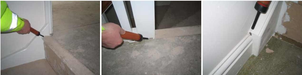
Figure 4.4 Gaps around the staircases.
