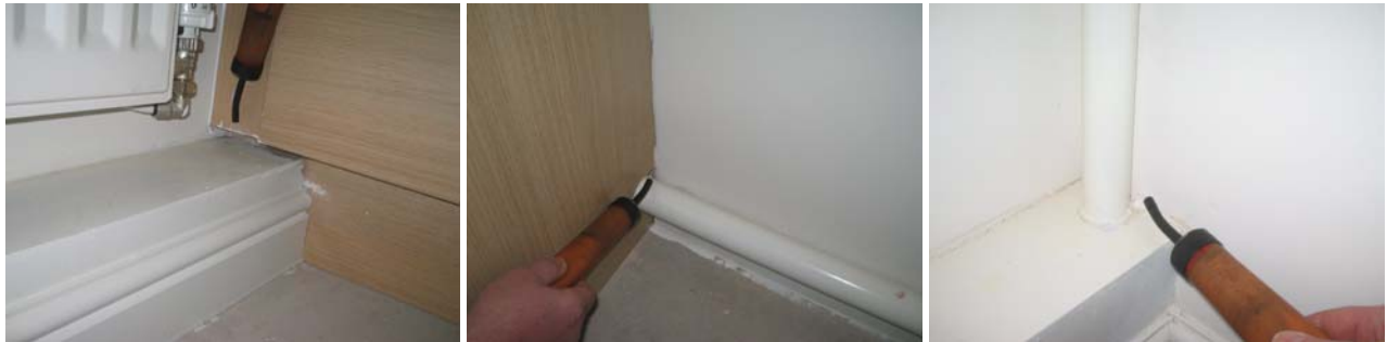
Figure 13.12 Increased air leakage at pipework boxing.
