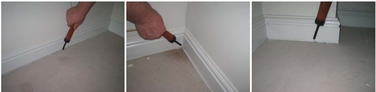
Figure 7.12 Air leakage in the lounge at the wall/floor junctions.
