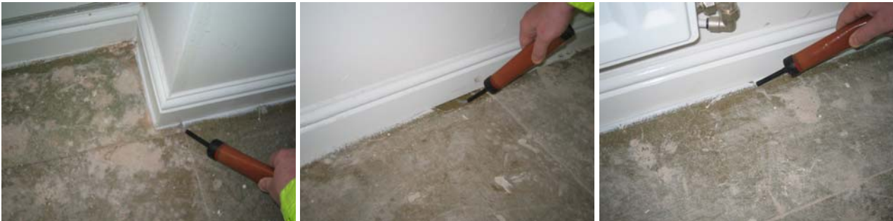
Figure 4.8 Air leakage at internal, separating and external wall/floor junctions on the second floor where gaps existed in the sealant.
