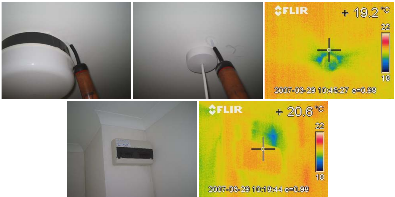
Figure 13.13 Air leakage around ceiling light fittings on the 2 nd floor, but still no leakage detected around the electrical consumer unit
