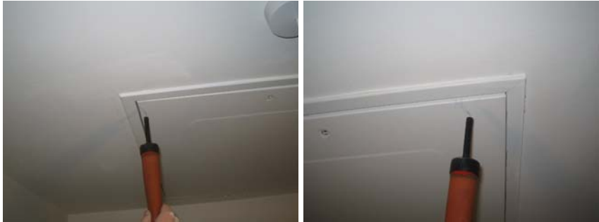
Figure 4.11 Air movement through the loft hatch.
