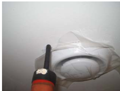
Figure 14.18 Air leakage around the vent for the MEV system in the kitchen.
