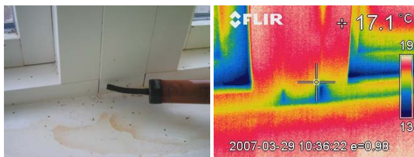
Figure 13.10 Direct air leakage gaps between individual frame elements of the bay window.
