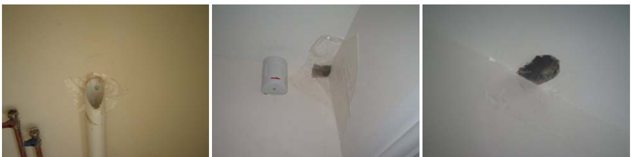
Figure 6.2 Temporary sealing to the washing machine waste pipe and to holes created during the installation of the security system.
