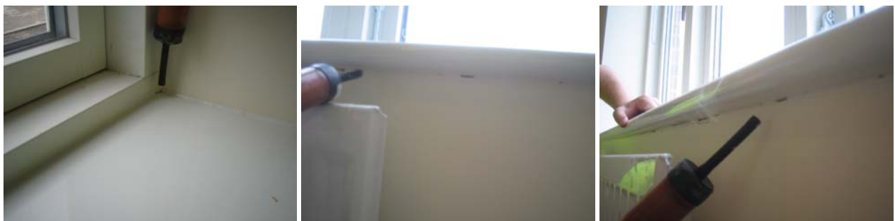
Figure 10.9 Air leakage detected around the window sills in the dining room and kitchen.
