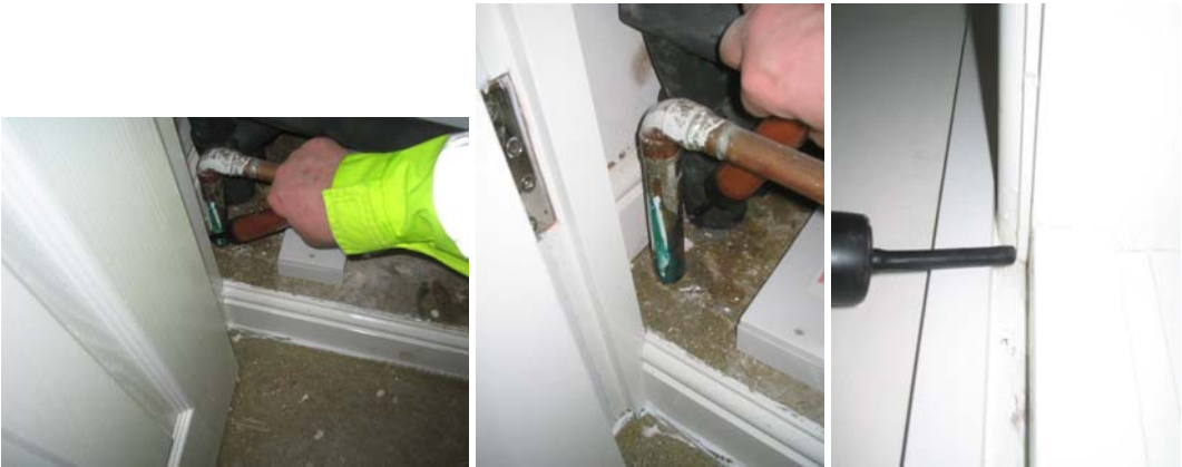
Figure 3.9 Air leakage in the cylinder cupboard.
