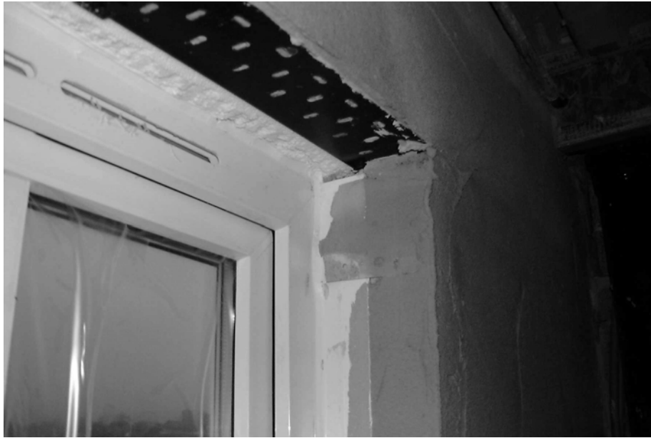
Figure 3 Gaps in parging at window reveals and underside of lintel
