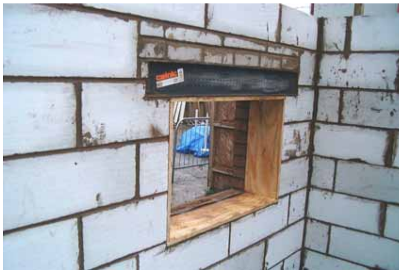
Figure 5: Test wall showing coursing problems caused by timber liner.
