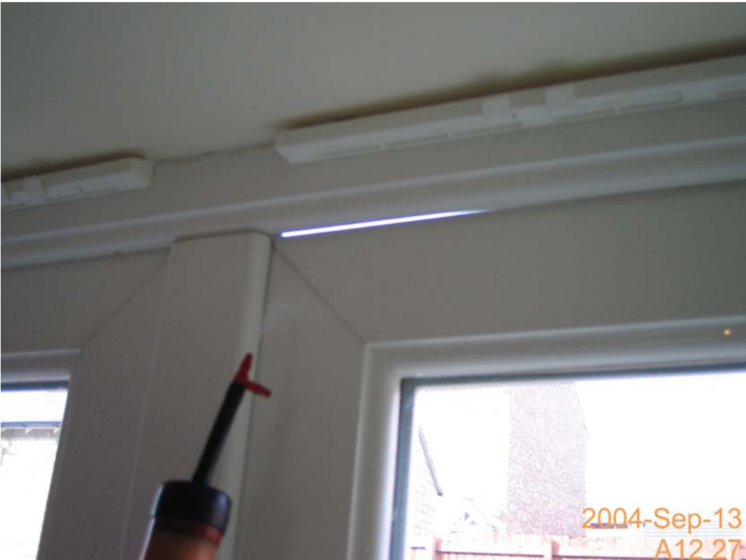
Figure 26 Poorly fitting patio door with visible gap.
