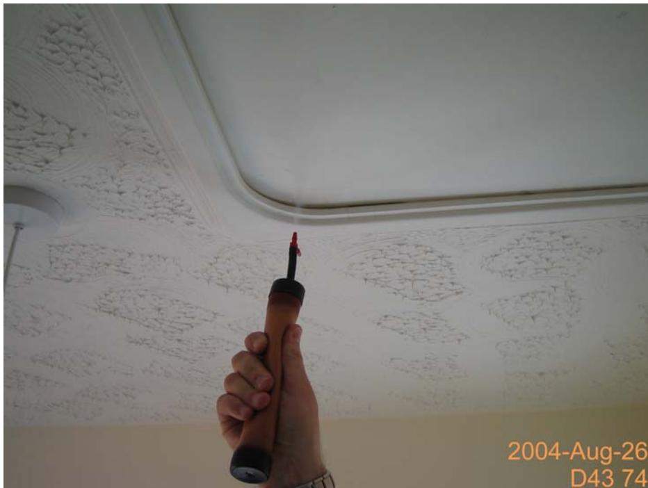
Figure 31 Leak through poorly sealed loft hatch.
