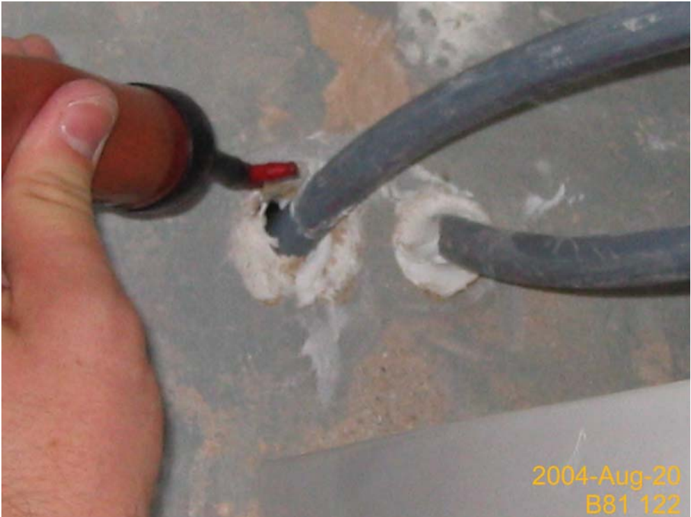
Figure 16 Unsuccessful attempt at sealing around water pipes.
