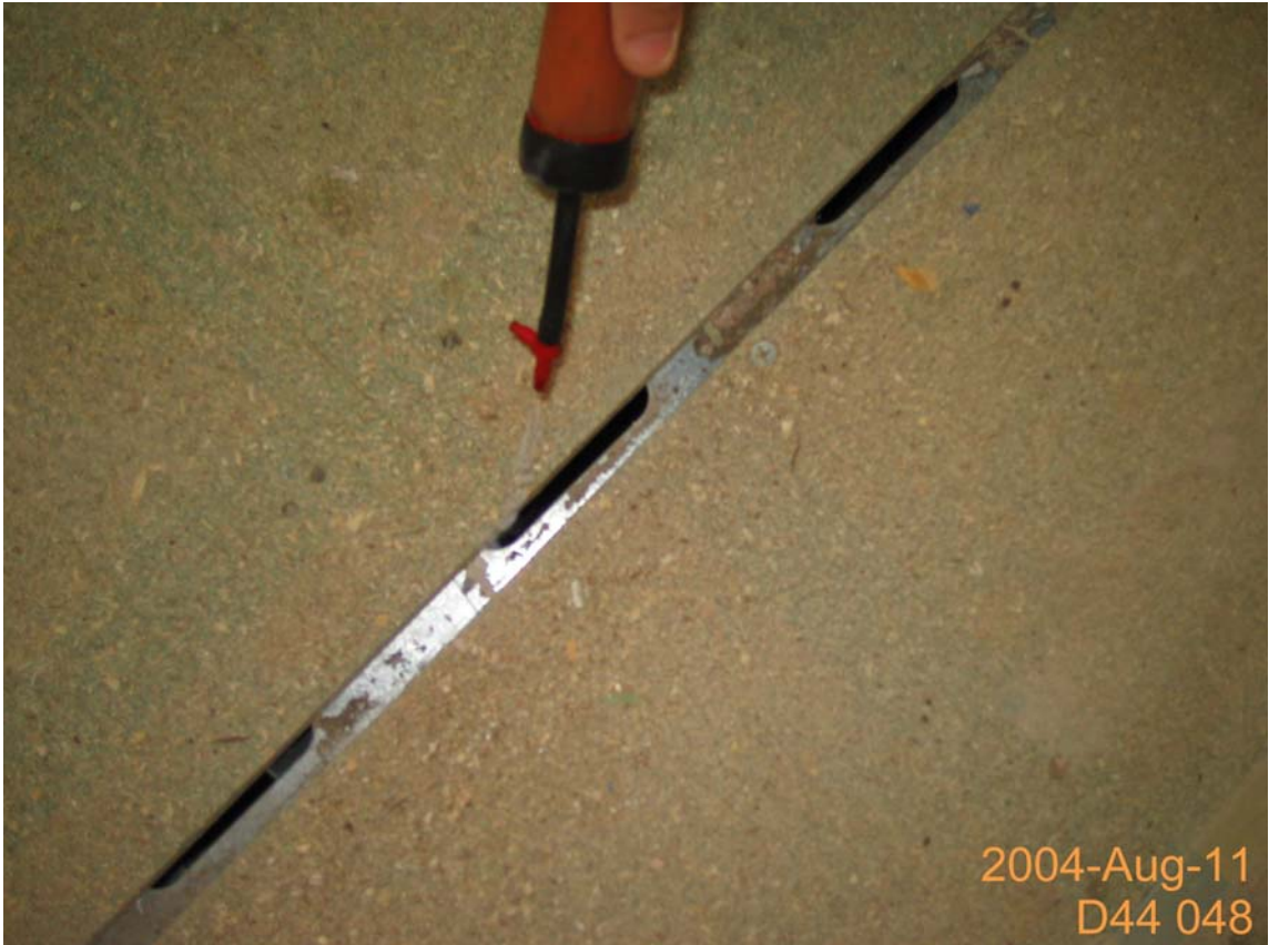
Figure 19 Leaks at the junction between flooring panels.
