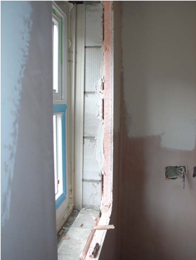
Figure 10 Discontinuous ribbons of adhesive around window opening.
