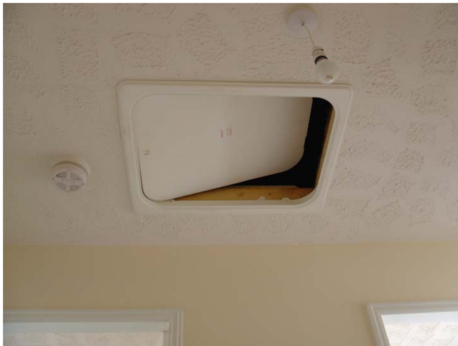
Figure 32 Loft hatch lifting during pressurisation test.
