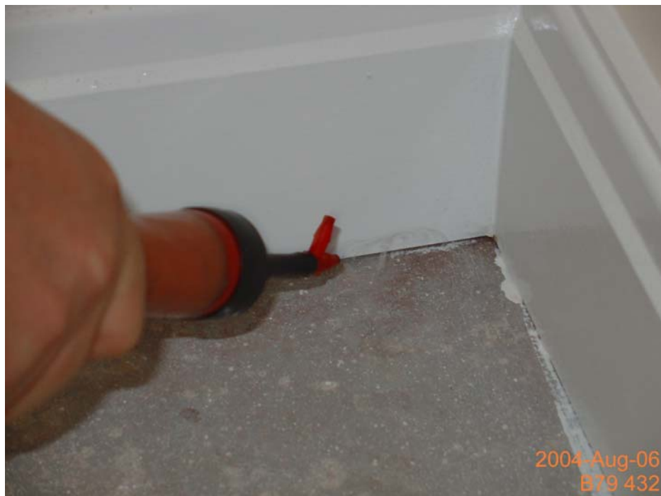
Figure 30 Gaps at the junction between the skirting board and the first floor.
