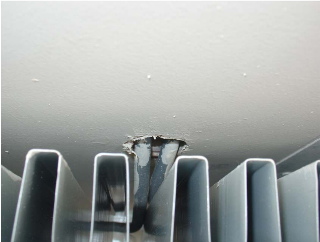
Figure 15 Unsealed pipework penetrations behind radiator.
