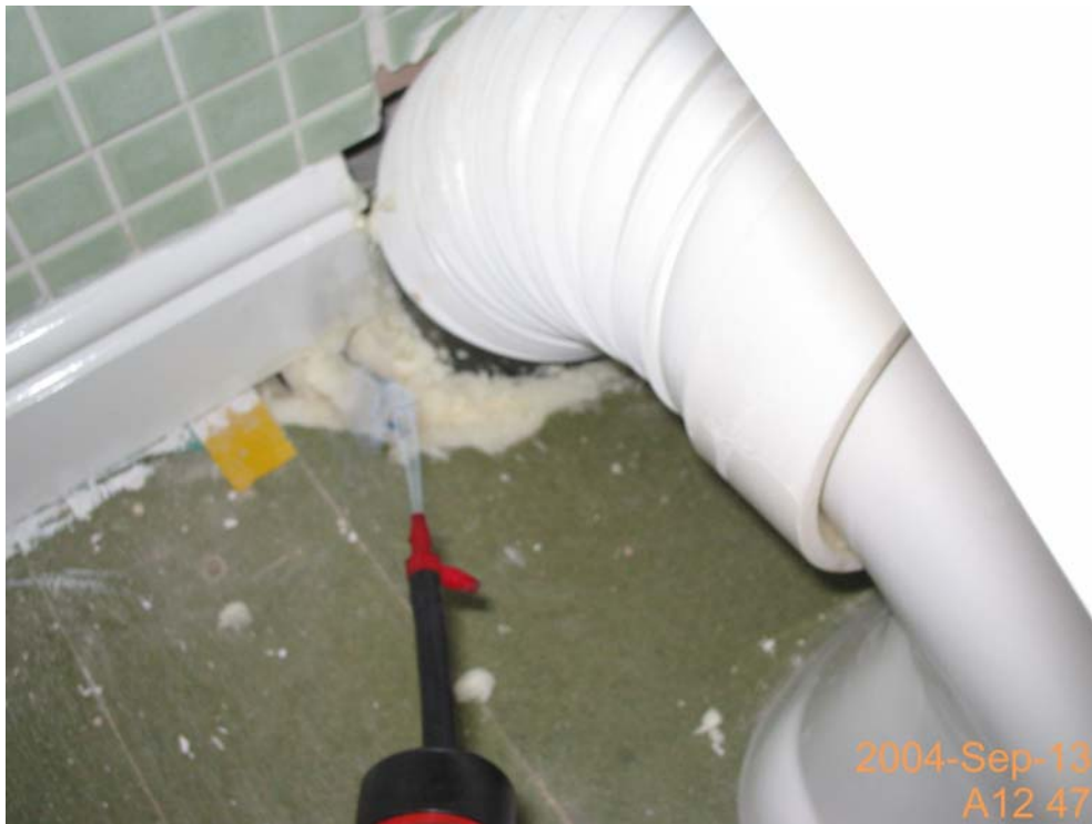
Figure 17 Inappropriate use of sealant to seal service penetrations.
