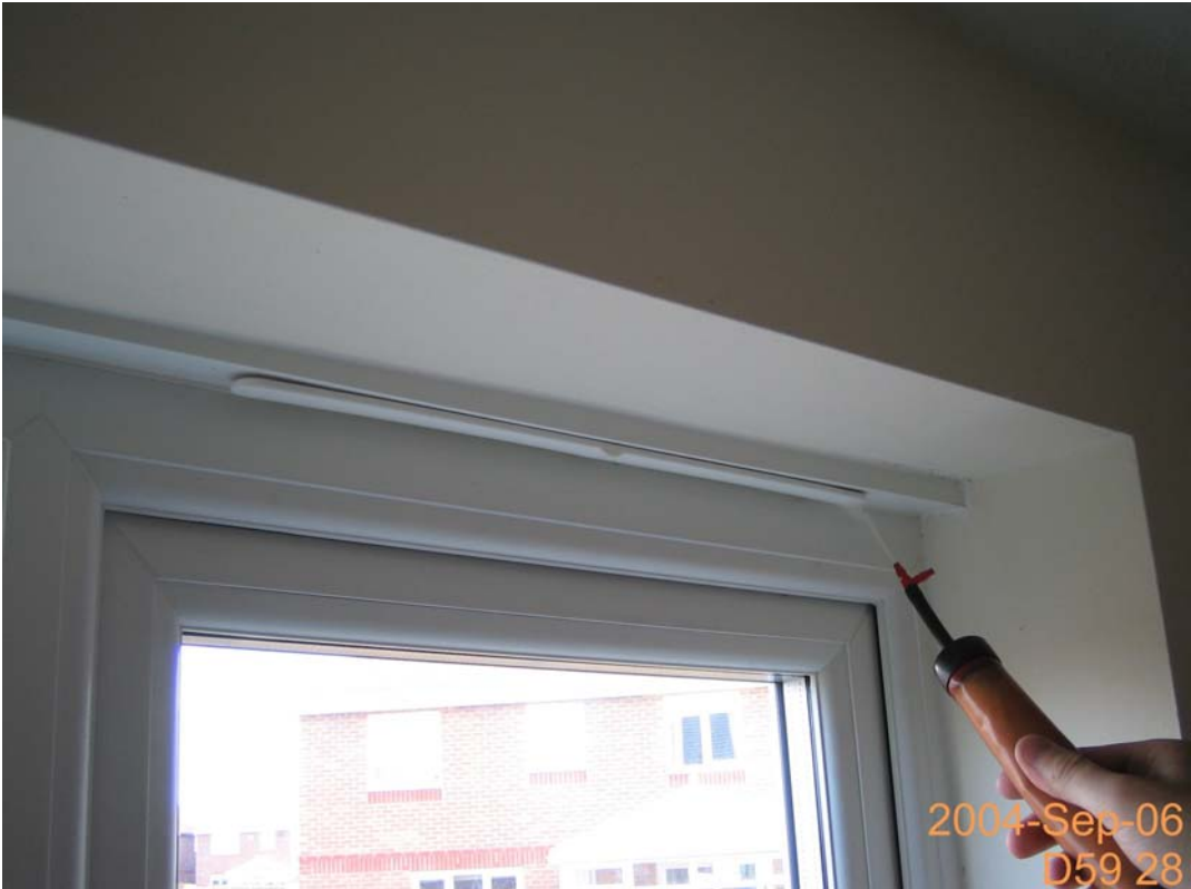
Figure 25 Leakage through poorly fitting trickle vents.
