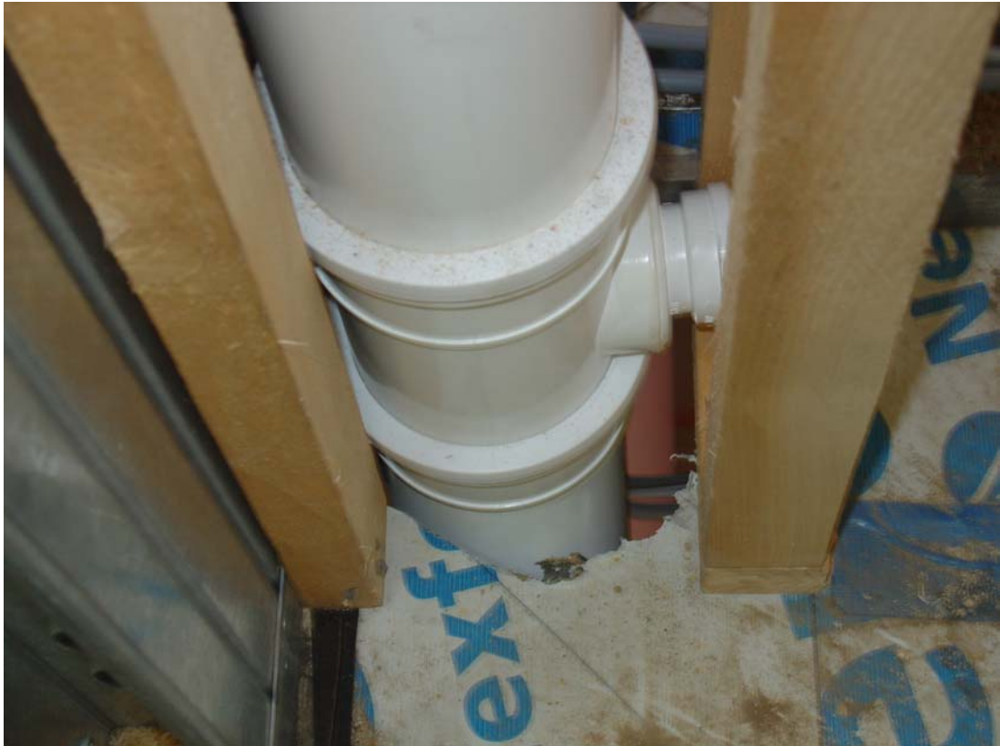
Figure 14 Unsealed soil stack penetrating through intermediate floor.
