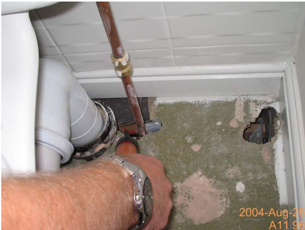
Figure 22 Holes in bathroom floor.
