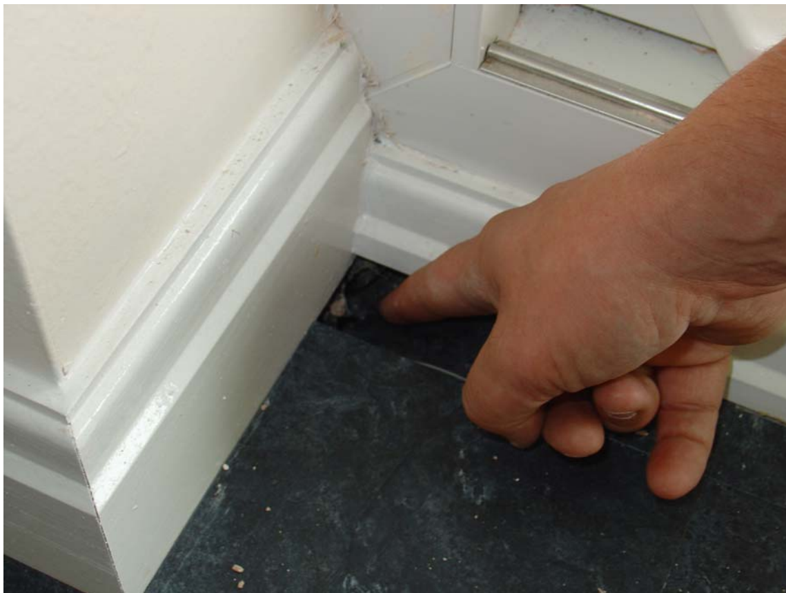
Figure 24 Hole in ground floor slab hidden by floor covering.
