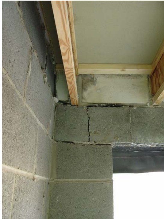
Figure 4 Cracks in internal blockwork leaf of external wall.
