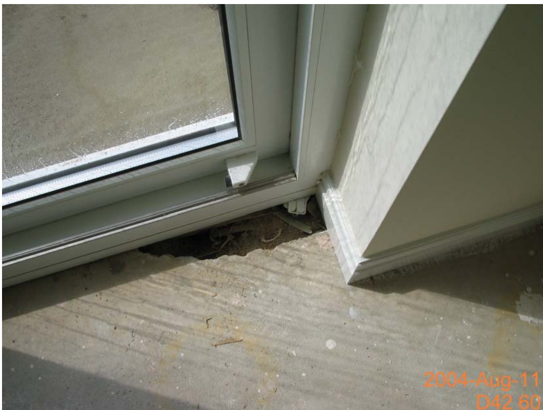
Figure 23 Hole in ground floor slab at patio door.
