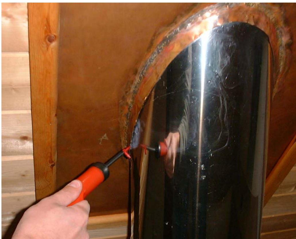
Figure B3 Leakage at the junction between the vent stack and the ceiling.
