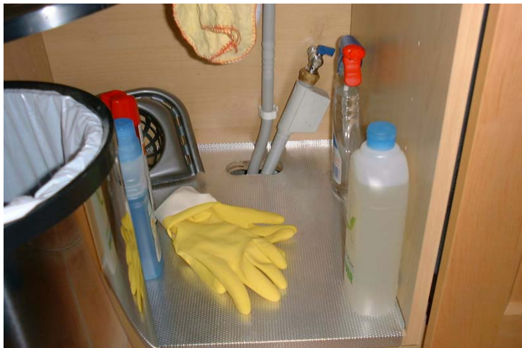
Figure B4 Leakage through service penetrations in the kitchen of Plot A.
