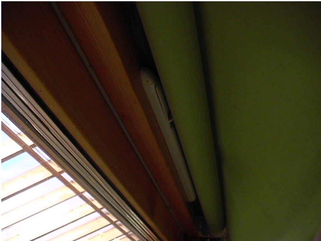
Figure B1 Leakage around trickle ventilator.
