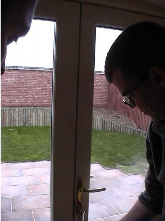
Figure B1 Leakage through opening casement of French door.
