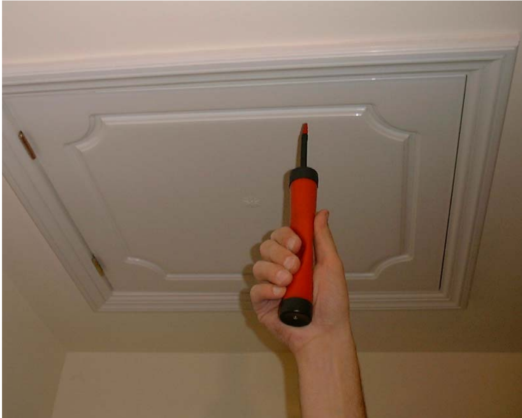
Figure B3 Leakage around the loft hatch.
