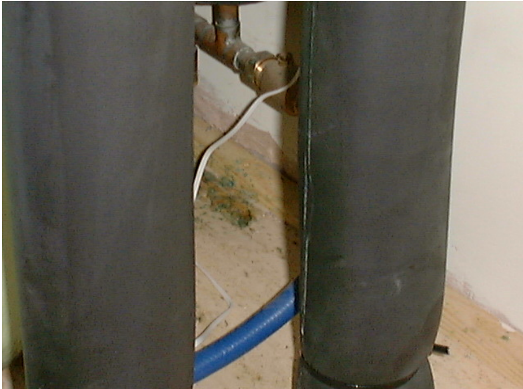
Figure B7 Leakage through service penetrations in the airing cupboard of Plot A.
