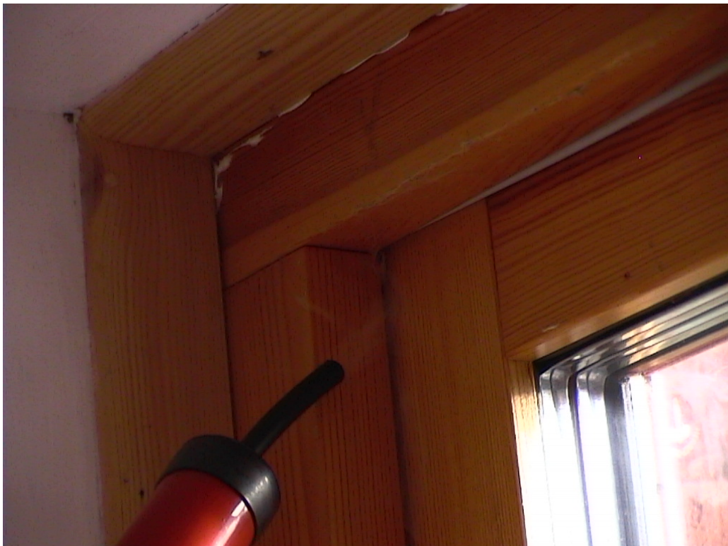
Figure B2 Leakage through opening casement of French door.
