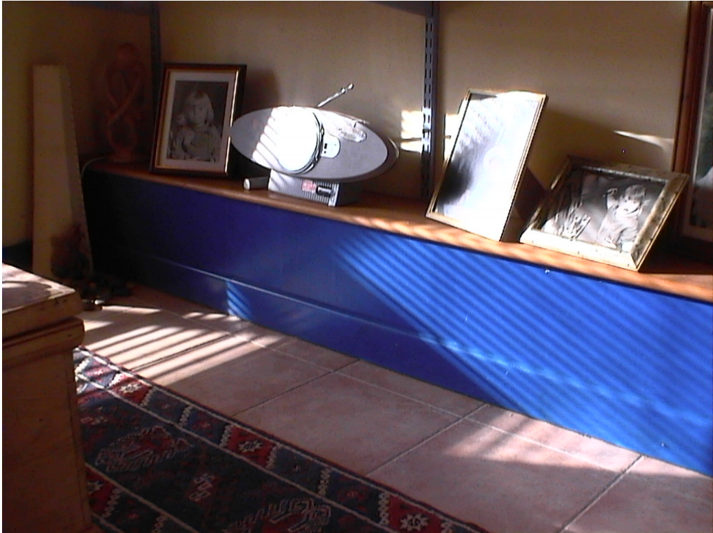
Figure B4 Leakage through boxed in services in the master bedroom.
