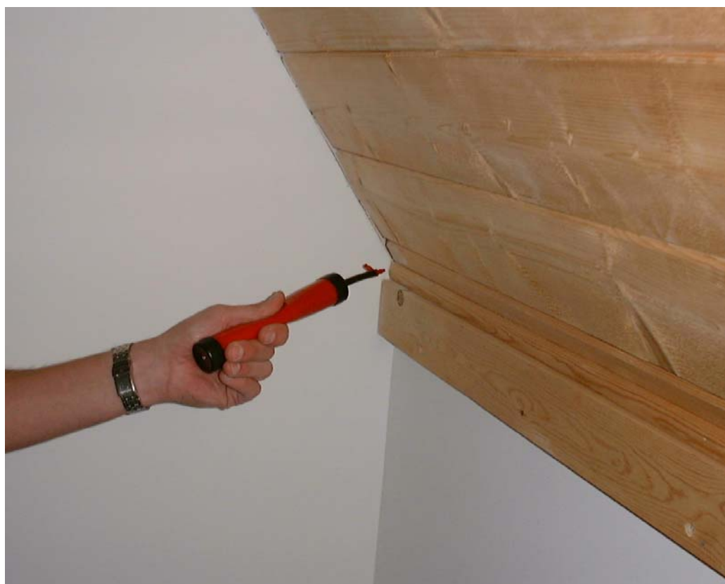
Figure B2 Leakage at junction between the ceiling and the internal and external walls.
