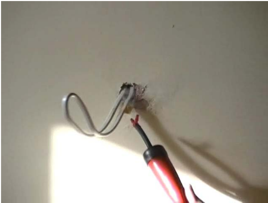
Figure B5 Leakage through exposed lighting loop in party wall.
