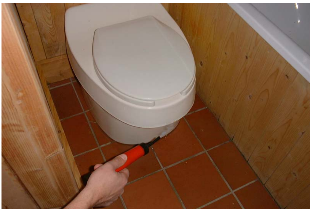
Figure B5 Leakage around the lid of the composting toilet.
