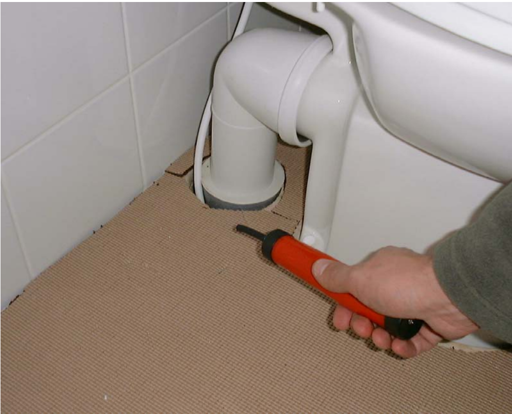
Figure B6 Leakage through service penetrations in the first floor bathroom of Plot A.
